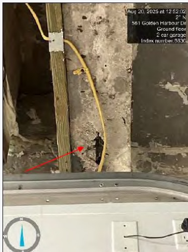
Crumbling concrete over exposed rusting rebar
