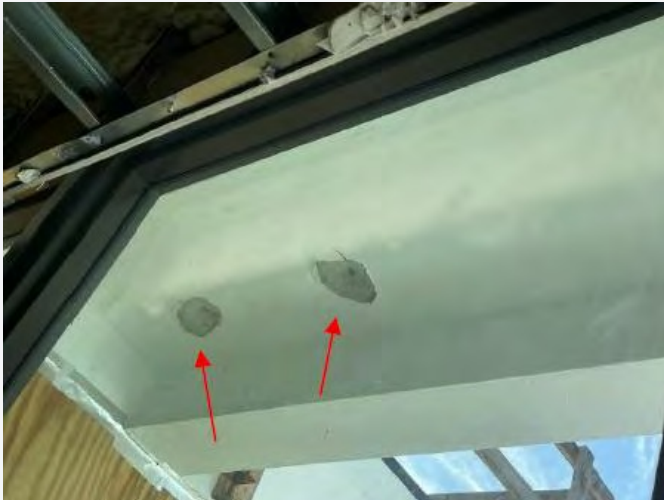
Holes drilled through balcony slab to drain ponding water — structural compromise
