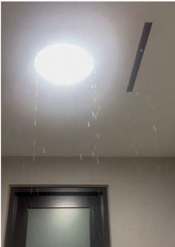
Water leaking from light fixture and AC diffuser — laundry room
