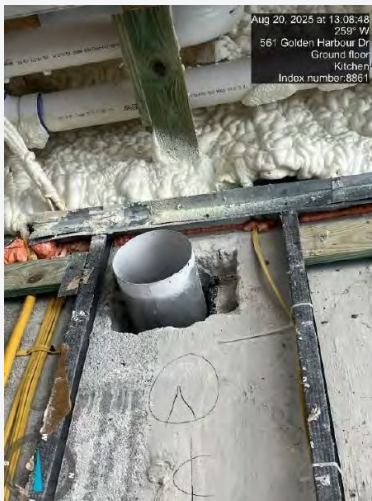
Kitchen air vent penetrating structural reinforced concrete column — critical code violation
