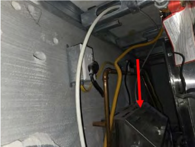
Steam generator behind gas cooking equipment — fire hazard
