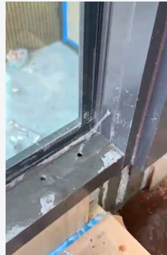
Water spouting from window frame — main staircase (after screw removal)
