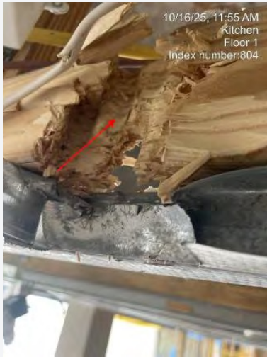
Broken roof trusses — trusses cut to pass vents and wires
