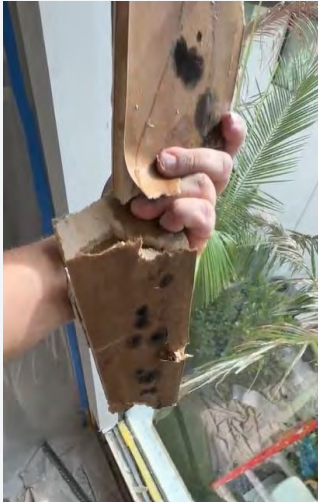
Black mold growing on drywall — daughter's room
