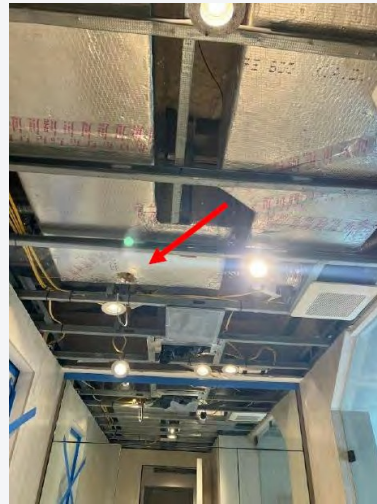
Hole drilled through HVAC air duct during light fixture installation
