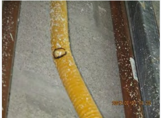
Screw hole through unprotected gas line — active gas leak
