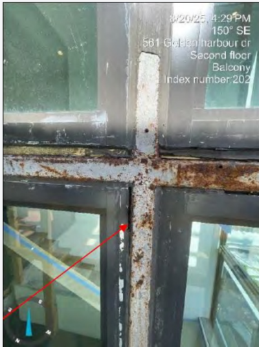
Corroded metal column and window mullion at main staircase with extensive water intrusion
