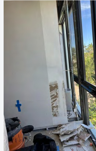
Water damage to children's rooms via window intrusion
