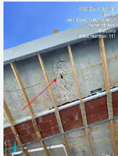
Honeycombing concrete on balcony slab — exposed rusting rebar
