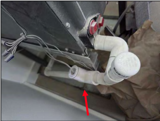
AHU #3 float switch in incorrect location
