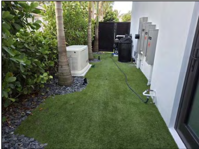
Emergency generator within near building opening
