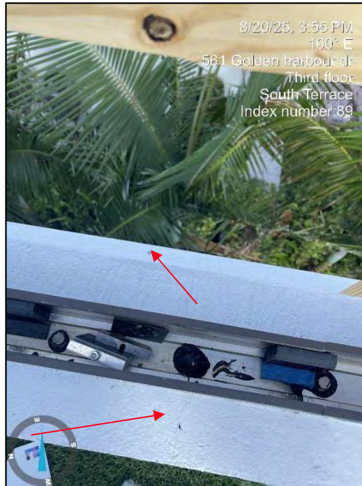
Photo 89 – Stucco crack at parapet wall adjacent to South Terrace of glass railing at Level 3.
