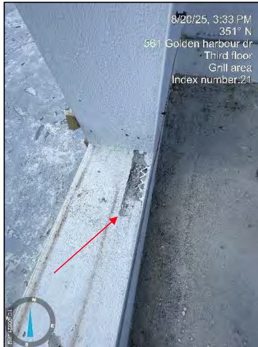
Photo 21 – Delaminated Stucco at parapet adjacent to Grill area at Level 3.
