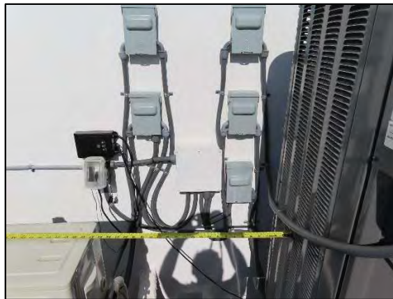
Condensing Unit Disconnects
