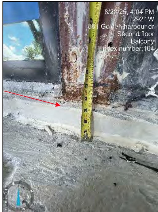
Photo 104 – Corroded metal column at master bedroom at the second floor.
