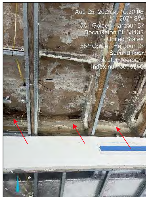
Photo 9246 – Water intrusion at the overhead beam in master bedroom at second floor.
