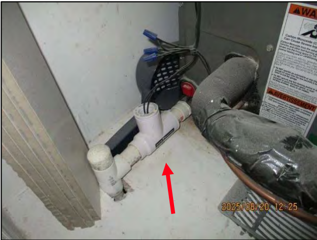
AHU #1 float switch in incorrect location
