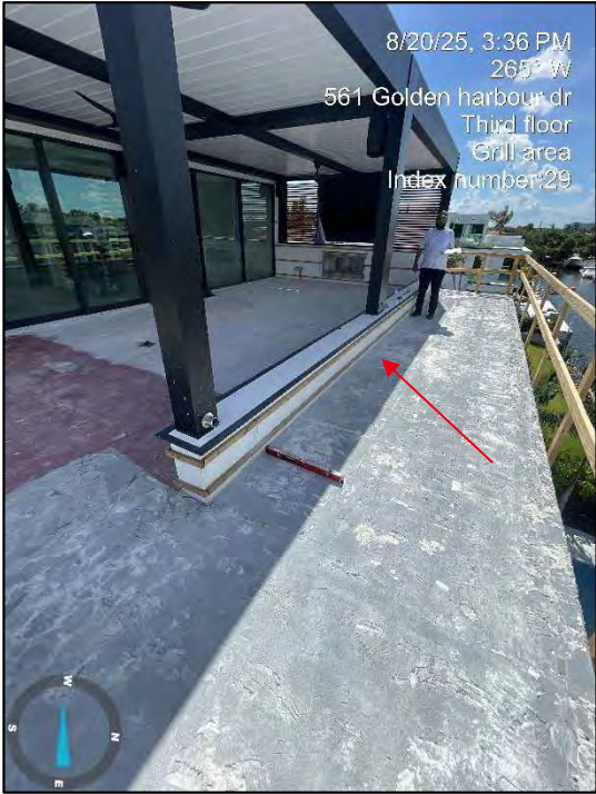
Photo 29: Emergency scupper not provided as per sheet P-03 at the curb on third-floor terrace.
