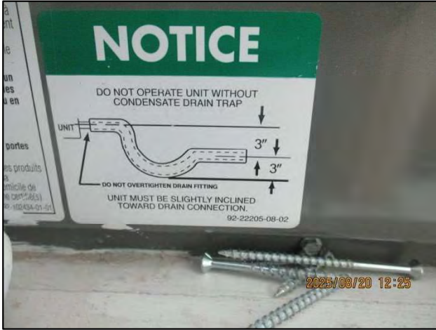
Label on AHU equipment indicates required trap.
