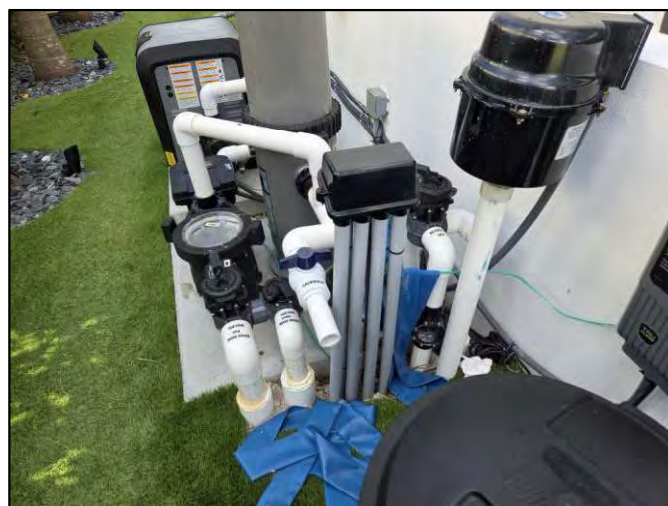
Exposed plastic PVC piping at the Pool/Spa equipment
