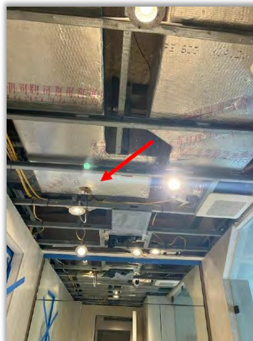
Figure 14: hole drilled through air duct due to light fixture installation
