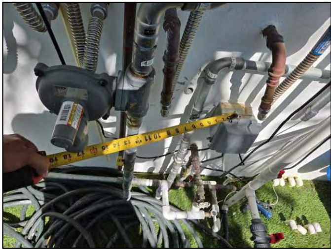
Water heater regulator within 3 feet of ignition source
