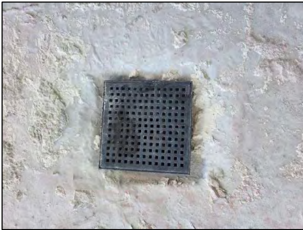
Typical grate/strainer installed at the outdoor Terrace.
