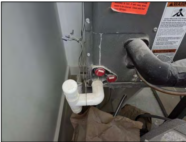
AHU #3 PVC condensate drain within return air plenum.
