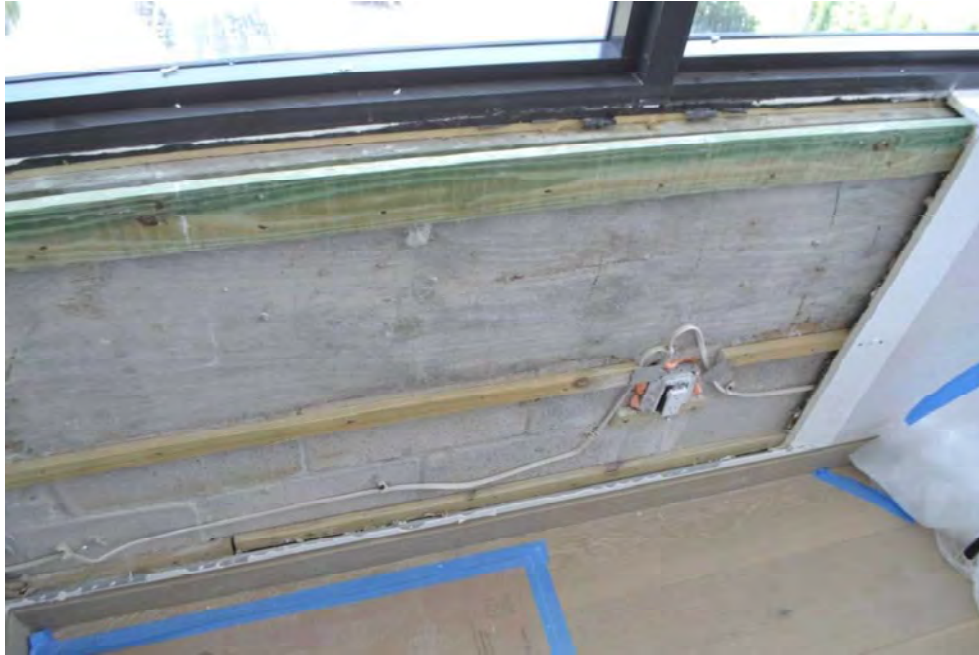
Figure 5) View of reported water damaged wall finish removed at the office.
