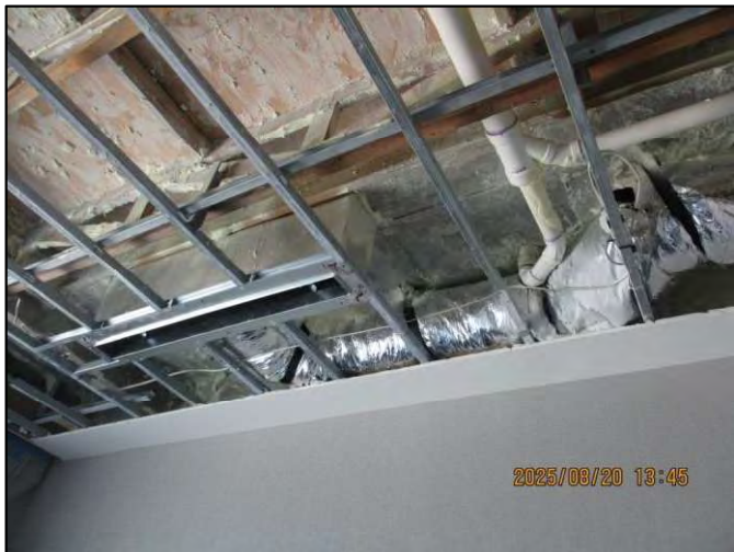
1 st Guest Bedroom with single SA duct where two are specified.
