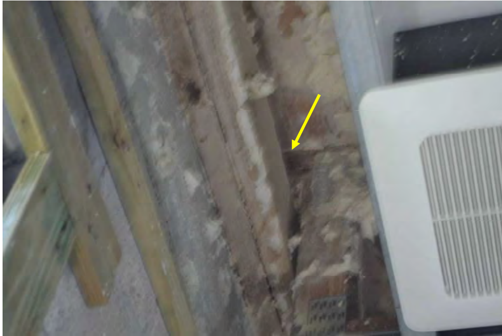
Figure 41) View of water staining observed to the floor framing above the daughter's bathroom.
