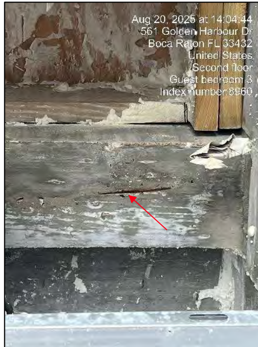
Photo 8960 – Corroded metal embedded in the beam at overhead ceiling of the guest bedroom #3 at second level.
