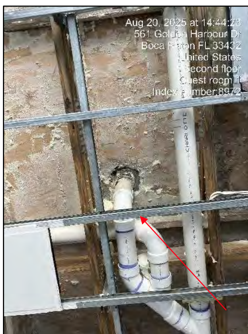
Photo 8972 – Signs of water intrusion adjacent to the pipe penetration at the overhead slab in guest bedroom #1 at second floor.
