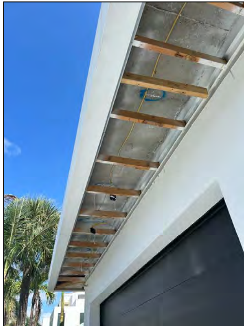
28 - Active leak location observed.
