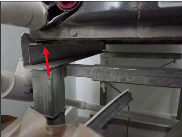
AHU #3 missing specified vibration isolator pads
