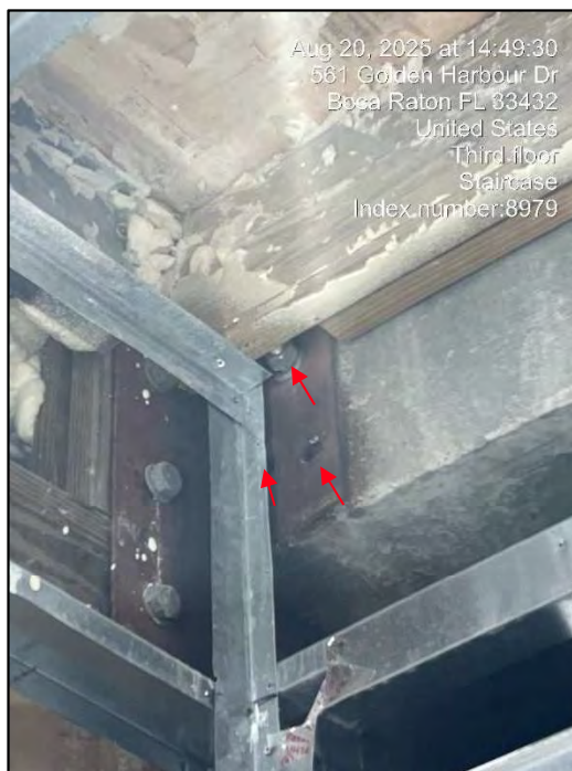
Photo 8979 – Missing bolts and a inclined installation of one bolt.
