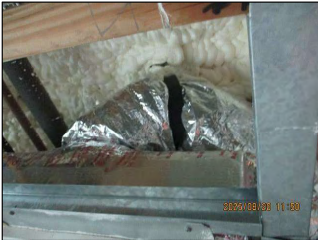
Typical condition of flexible ducts with sharp bends and compressed insulation at vent box connection, Laundry Room.
