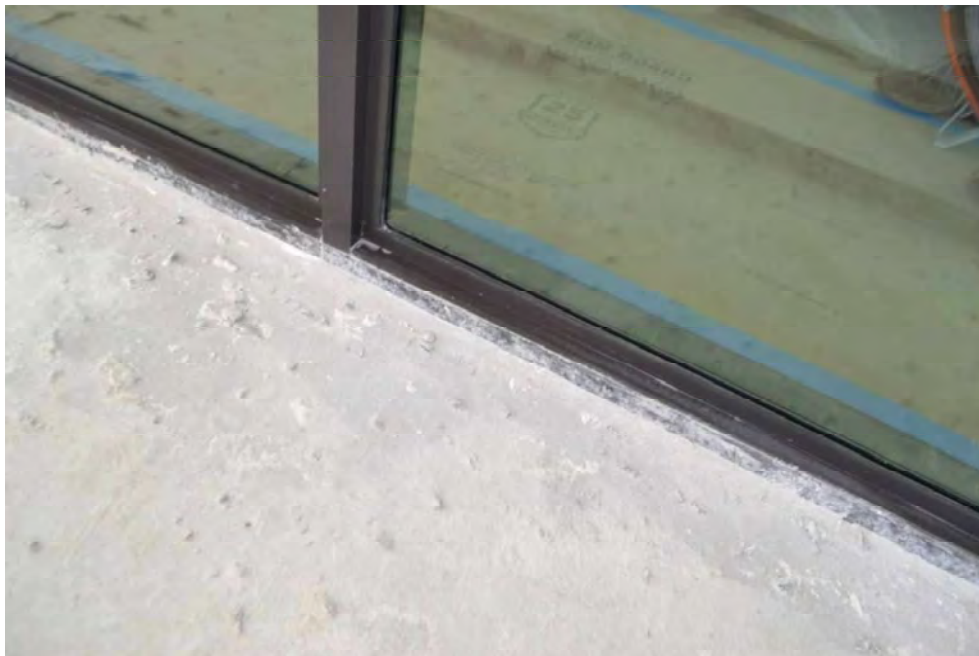
Figure 16) Exemplar view of removed pavers at the third floor rear balcony. Note pavers installed above lower window frame in some locations.
