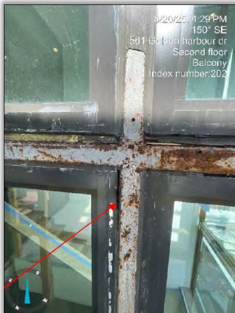
Figure 9: corroded metal column and window mullion at main staircase with excessive water intrusion
