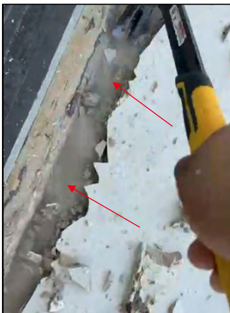
Photo 561 – 6.9.25 – Video #2 Still: Second Floor Balcony – Showing water standing below floor finishes during demolition adjacent to window wall.
