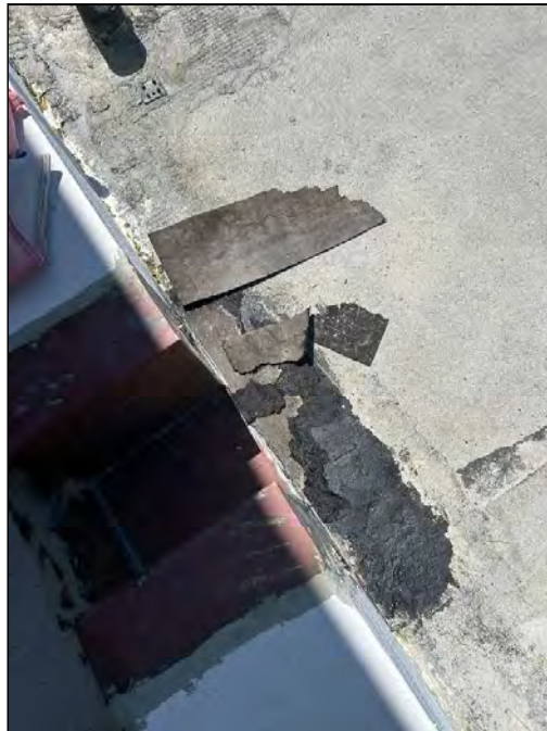
14 - Membrane repair not properly adhered to substrate.
