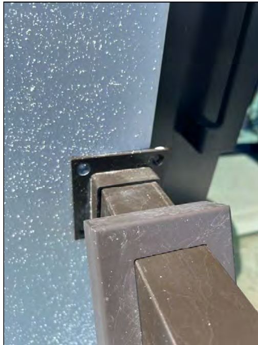
24 - Missing fastening screws, exterior wall system unsealed.
