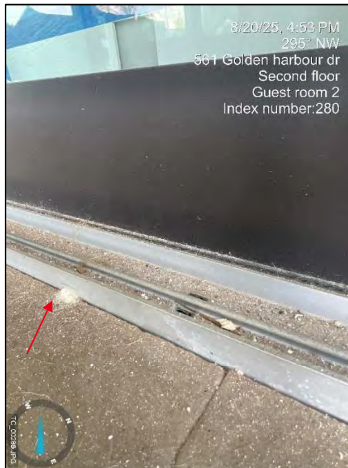
Photo 280: Signs of galvanic reaction and pitting at contact with tile finishes/mortar system at the ground floor outdoor living area adjacent to the dining room.
