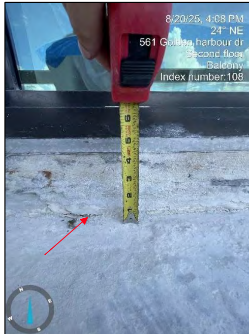
Photo 108 – Sliding glass door with excessive gap between framing and structural substrate at sill at second level balcony.
