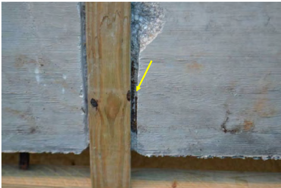
Figure 56) View of exposed reinforcing observed at the removed concrete at a beam at the ceiling furring strips above the rear porch.
