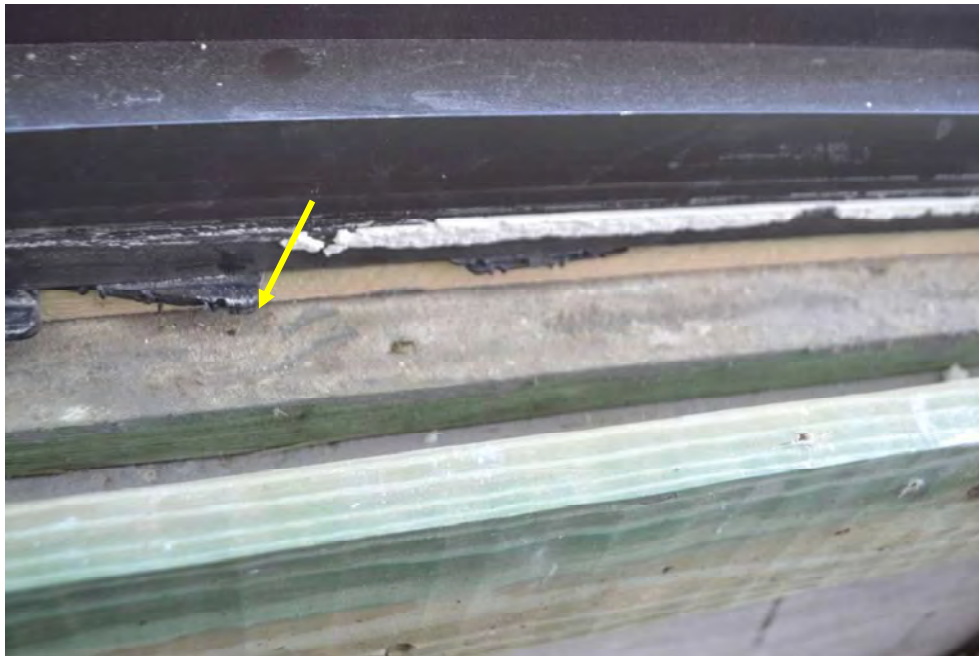
Figure 6) View of water staining observed to the window buck in the office.
