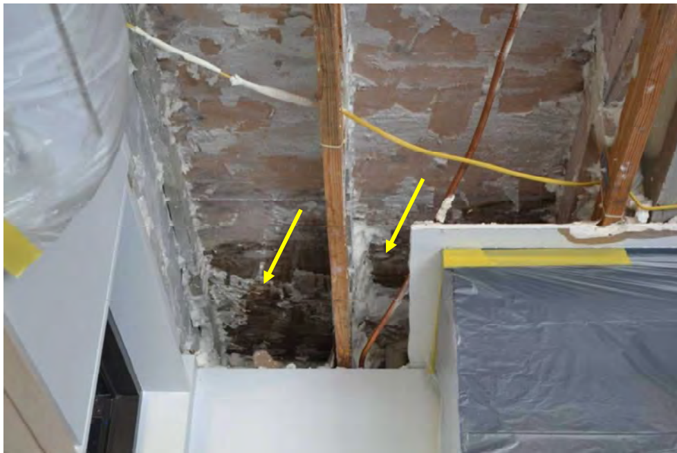
Figure 52) View of water damage and deterioration observed to the floor sheathing above the garage.
