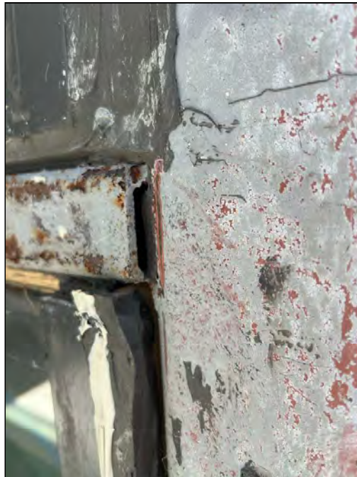
6 - Window assembly observed without proper sealant.
