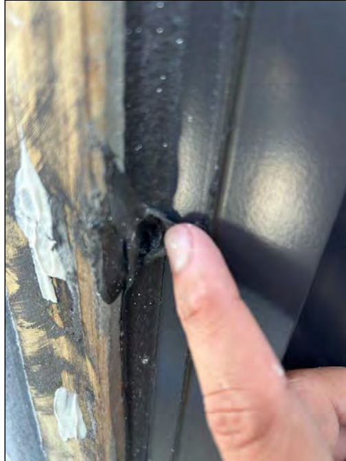
23 - Inconsistent application of sealant at window perimeters
