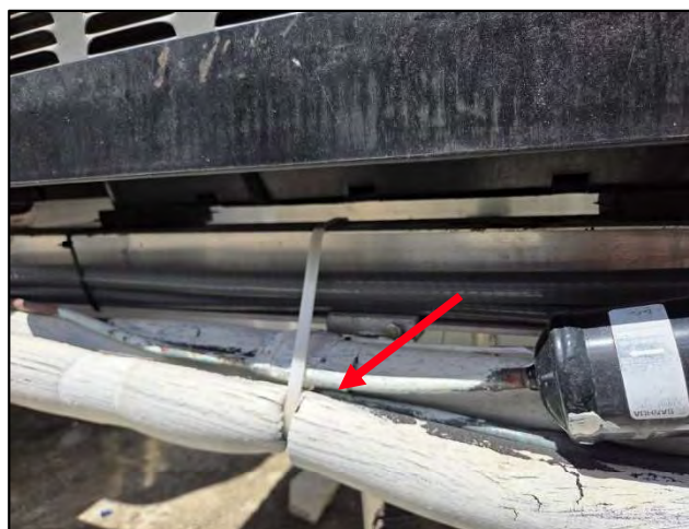
Typical conditions of zip ties supporting refrigerant piping and compressing insulation
