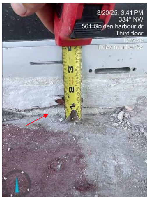
Photo 62 – Sliding glass door with excessive gap between framing and structural substrate at sill at third level terrace.
