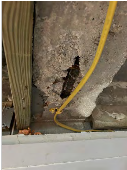
8 - Active leak observed during visit.
