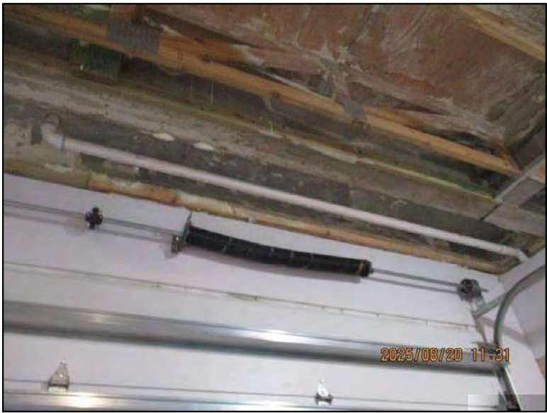
Piping hangers missing to properly support the piping
