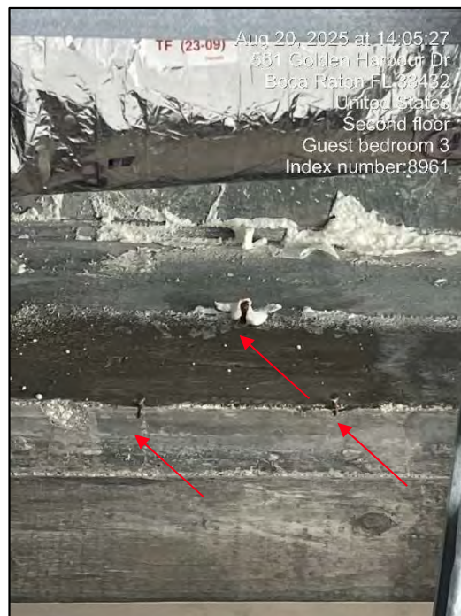
Photo 8961 – Corroded metal nails embedded in the beam at overhead ceiling of the guest bedroom #3 at second level.
