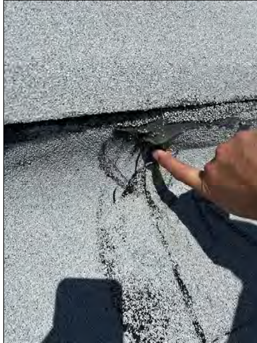
1 - Hole observed at the roof membrane to be detailed.
