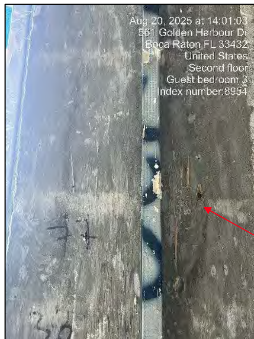
Photo 8954 – Corrosion stain visible at wall in Guest bedroom #3 at the 2 nd Floor.
