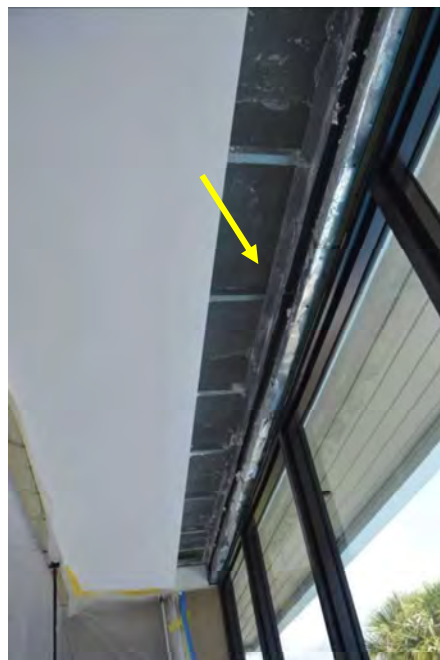
Figure 38) View showing the reportedly water damaged ceiling finish removed in the master bedroom along the exterior windows.
