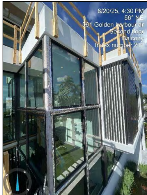
Photo 211 – Corroded metal columns and horizontal members at staircase landing at the second floor.
