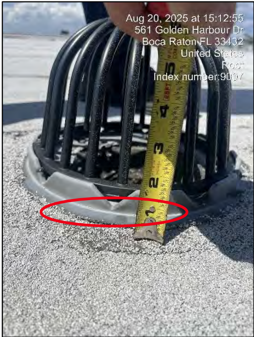
Photo 9007: View of roof drain at 4 th Floor. Note the drain is installed above the Roofing System.
