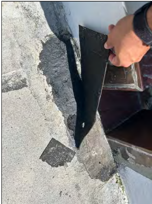
18 - Roofing membrane repair loose.
