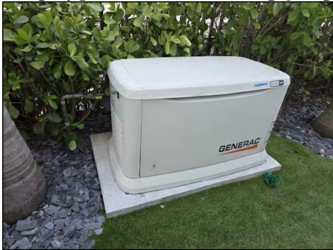
Trees installed within 3 feet of generator
