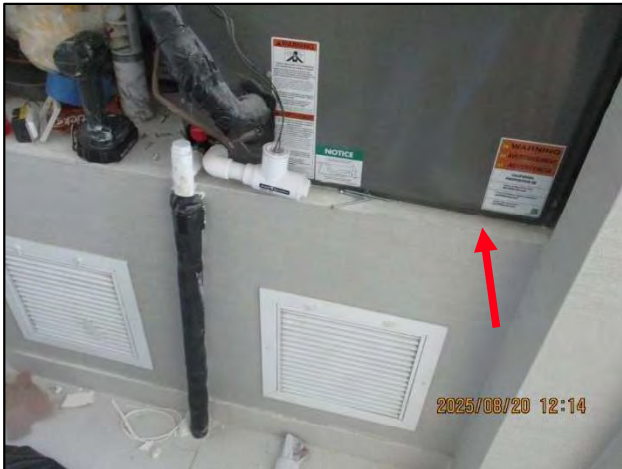
AHU #2 missing specified vibration isolator pads
