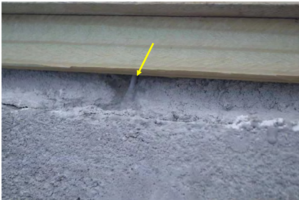
Figure 12) Close-up view of low-strength grout installed between the window buck and concrete beam at the stair to the third floor. Note window anchor.
