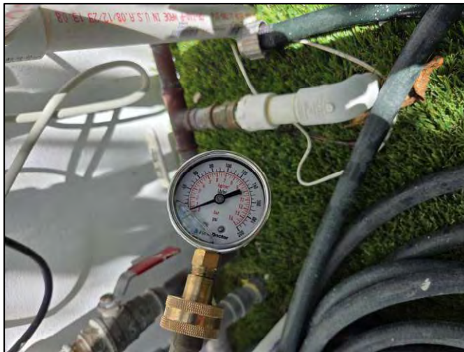
Domestic water supply pressure drops to near zero when irrigation system is operating.
