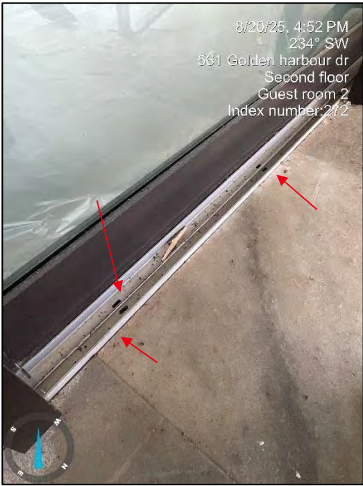
Photo 272: Tile covering the weep holes at aluminum glazing frame and in contact with sliding glass door frame at the first floor.
