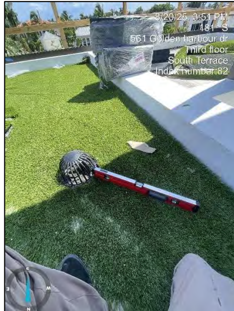
Photo 82: The slope of the roof is away from the drain -East Terrace at 3rd Floor.
