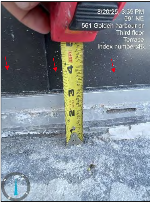
Photo 48: Stains on the aluminum frame show the level of tile and mortar bed prior to removal of tiles. It is evident that the weep holes were blocked by tile and mortar system at the third-floor terrace.
