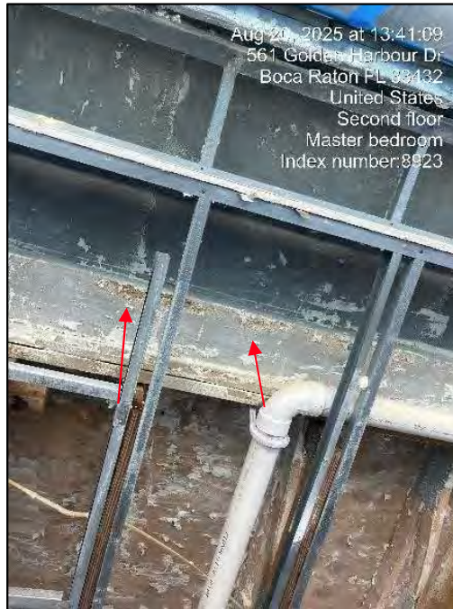
Photo 8923 – Water intrusion at the overhead beam in master bedroom at second floor.
