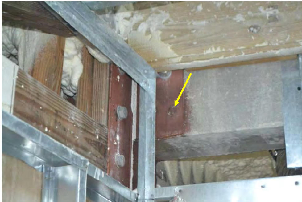
Figure 8) View of a missing anchor at a girder truss connection above the stair to the third floor.
