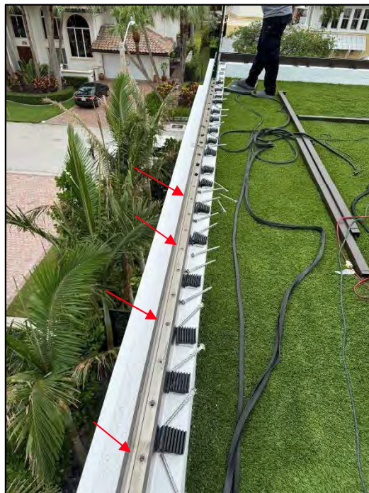
561-6.5.25-Pic #14 – Fasteners at the base of railing system were not provided with sealant.
