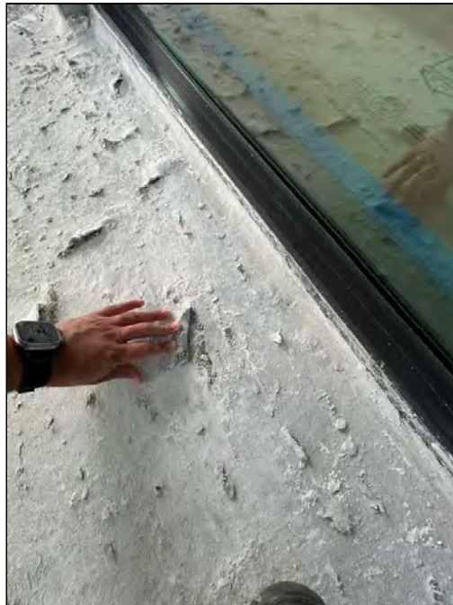
20 - Waterproofing system not adhered to substrate.
