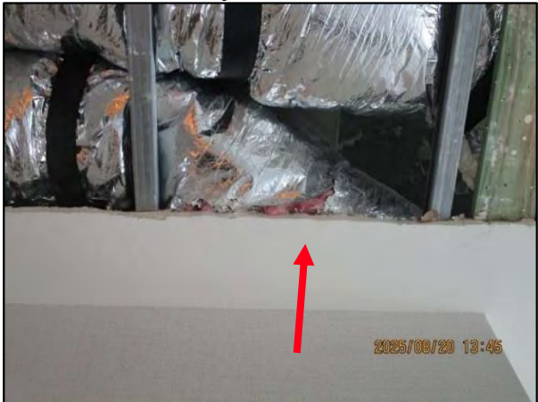
Typical condition laceration observed in duct insulation, Bedroom 3.
