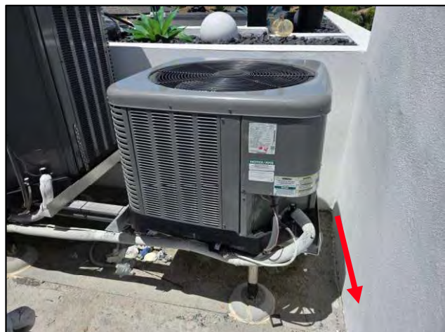
Emergency overflow drain missing at the Mechanical Roof Area
