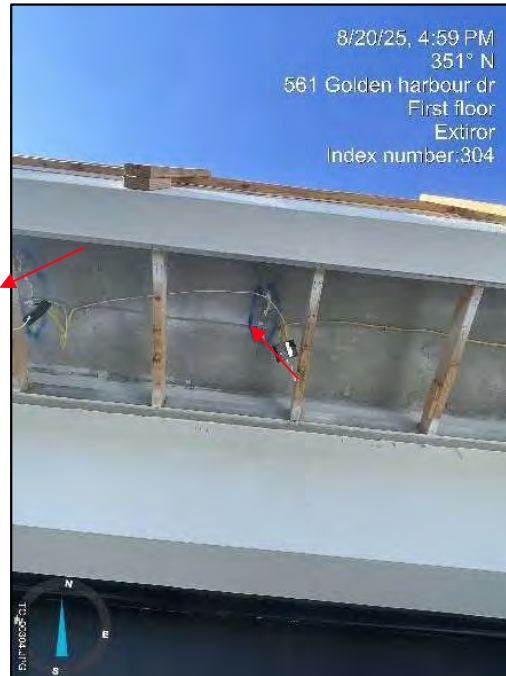
Photo 304 – Multiple cracks at the concrete ceiling slab at the Southwest corner of the office – 2 nd level.
