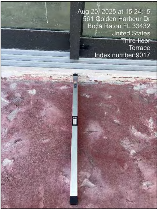
Photo 9017: Third Floor Terrace – General view of the north terrace without any slope. Client has reported water intrusion from this area damaging the interior floor finishes.
