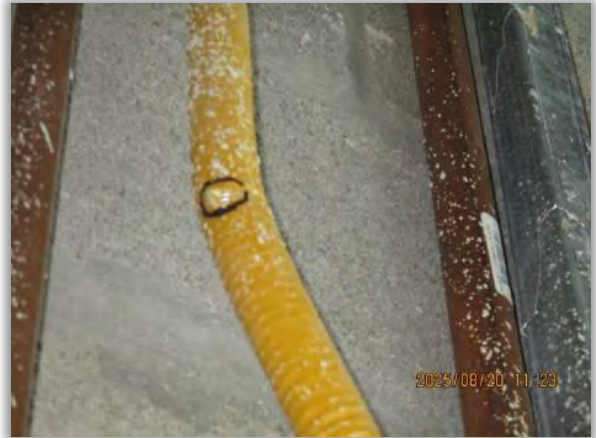
Figure 16: screw hole in unprotected gas line
