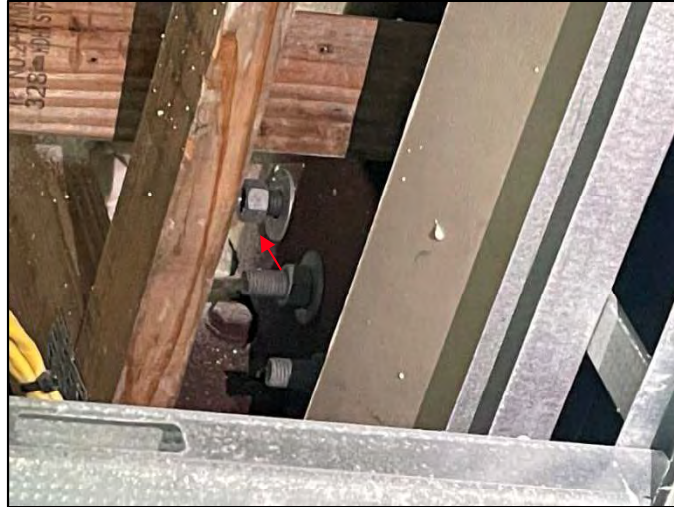
Photo 5560 – Loose bolts at his bathroom at level 2 (west).
