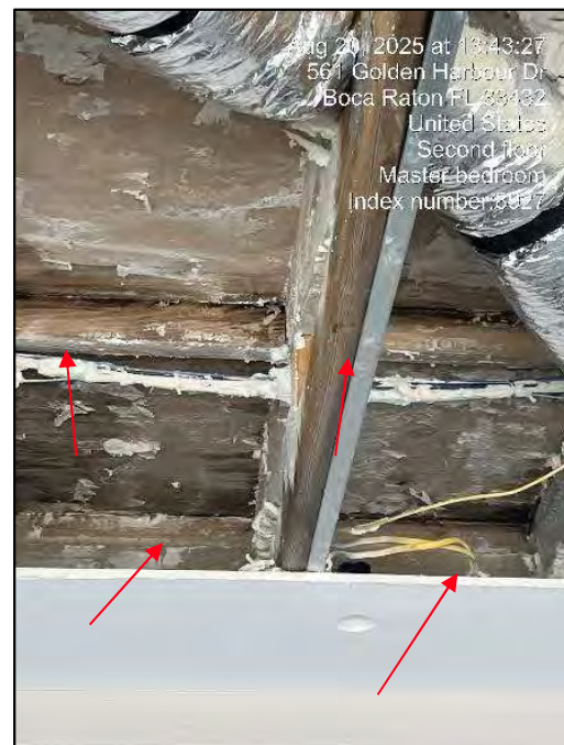
Photo 8027 – Water intrusion from the overhead slab in master bedroom at second floor.
