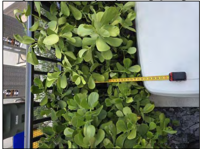
Fence installed within 3 feet of generator and bushes installed up against generator
