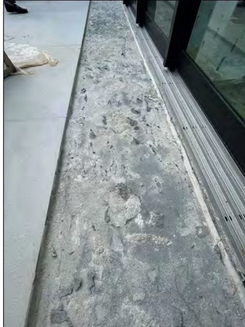
15 - Level 3 Balcony - Damaged waterproofing membrane.
