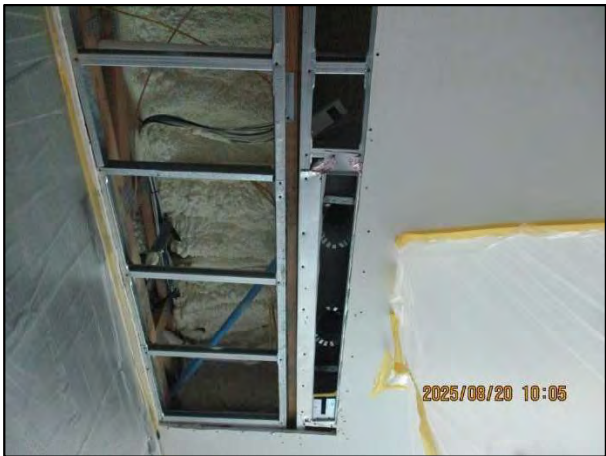
Air diffuser in the Dining Room
