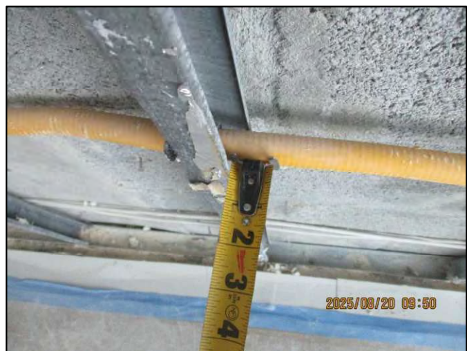
Installation of the CSST missing protection shield at the Kitchen wall
