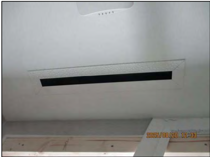
Condensation at diffuser in Laundry Room
