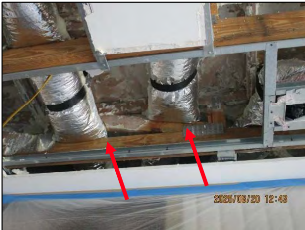
Typical condition of flexible ducts squeezed between floor beams and joists, Master Bedroom.
