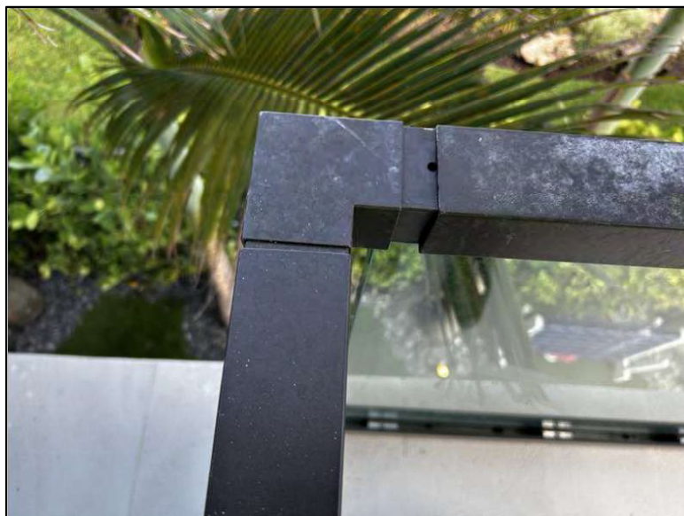
ECS Photo – Unsecured balcony railing system cap components.
