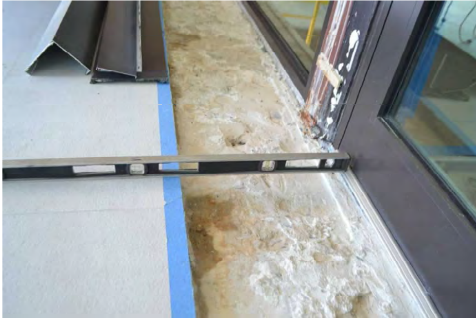
Figure 31) View showing pavers installed at or above the door threshold at the second floor rear balcony.
