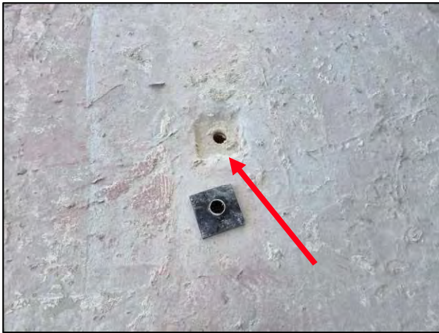
No drain body or clamping collar assembly installed for the Terrace drains.
