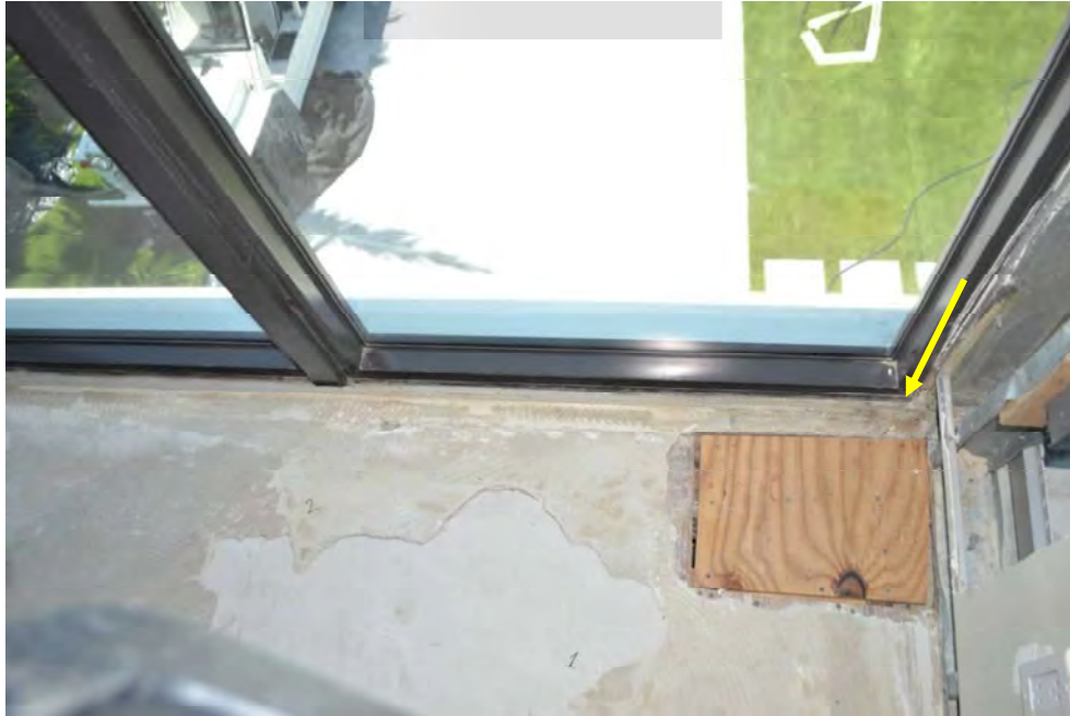
Figure 43) View of water staining observed to the concrete in the daughter's bedroom.
