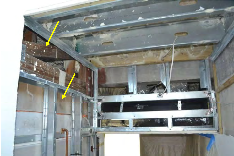
Figure 9) View of water damage and/or apparent fungal growth observed to the wall finish and truss at the stair to the third floor.
