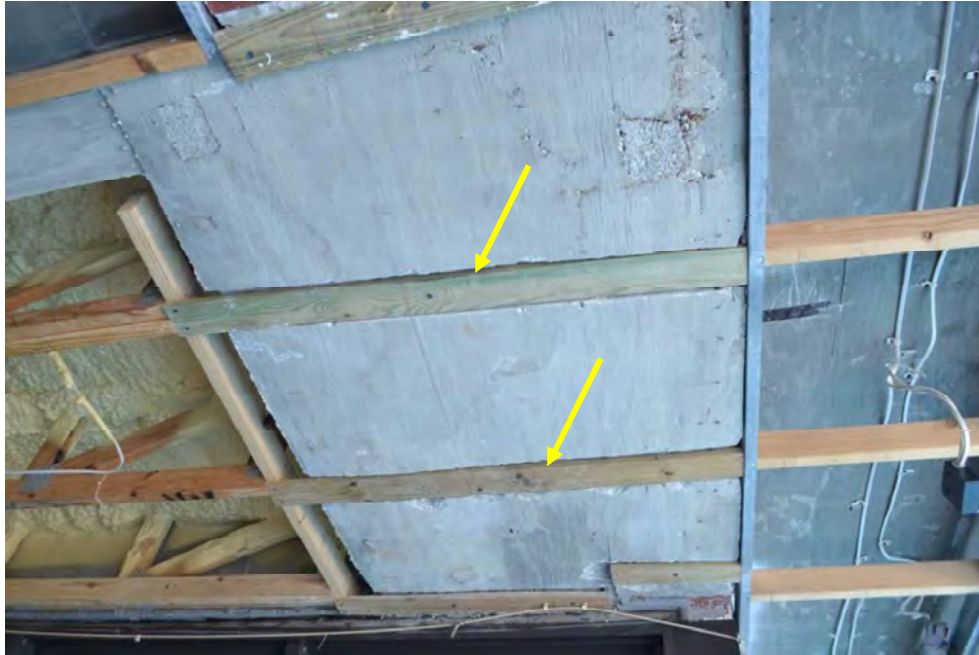
Figure 55) View of removed concrete at a beam at the ceiling furring strips above the rear porch.
