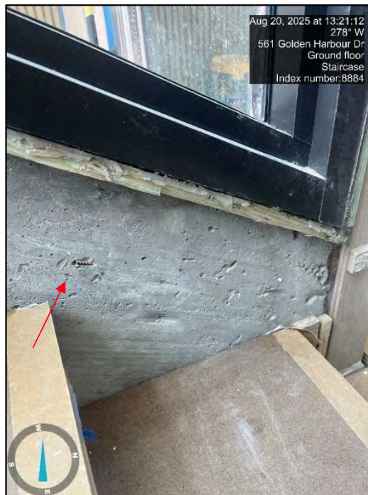
Photo 8884 - Exposed corroded nail at the staircase landing at the first floor.
