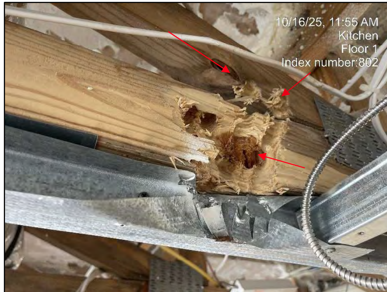
Photo TC_00802 – Damaged/broken truss member is visible at kitchen at Level-2.
