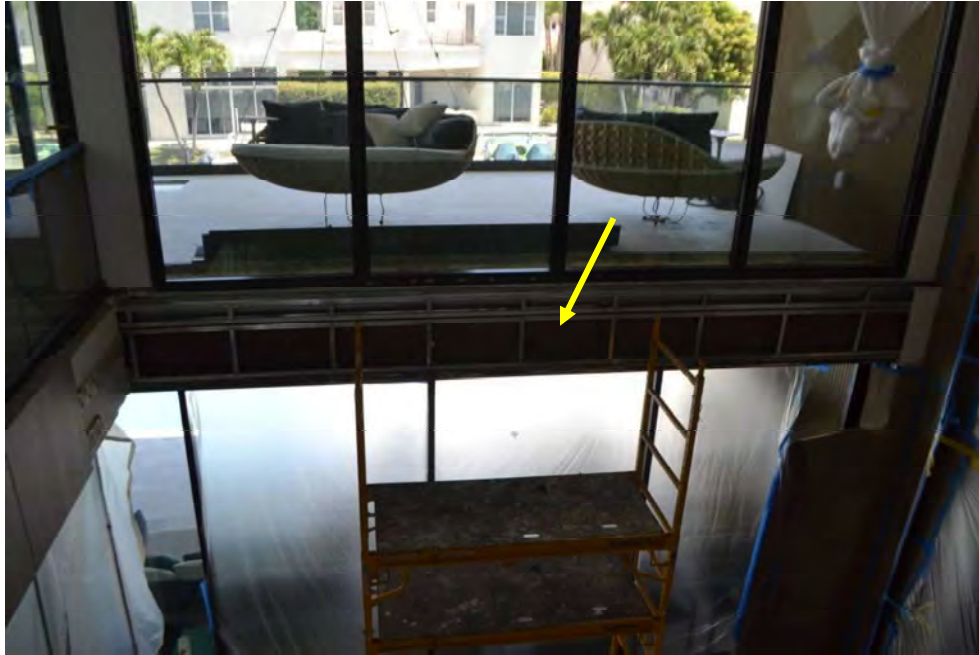
Figure 39) View showing the reportedly water damaged wall finish removed in the family room below the exterior windows.
