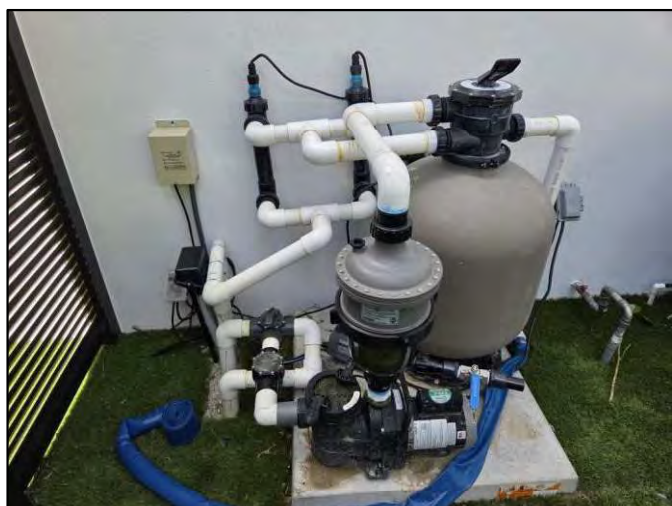
Exposed plastic PVC piping at the Koi Pond equipment
