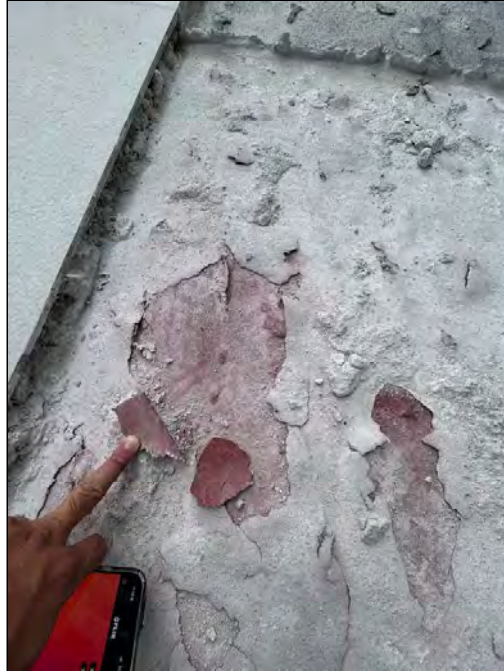
21 - Multiple layer of waterproofing material without clear indication of compatibility.
