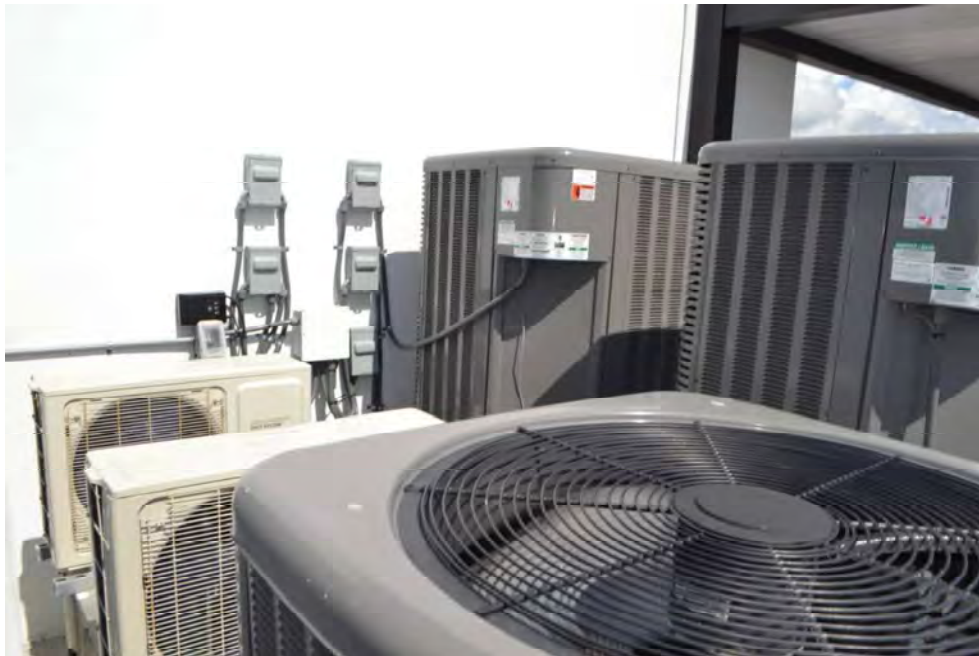
Figure 18) Overview of the outdoor mechanical area.
