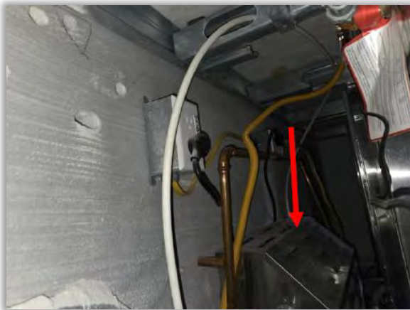
Figure 17: steam generator equipment installed behind gas cooking equipment; fire hazard
