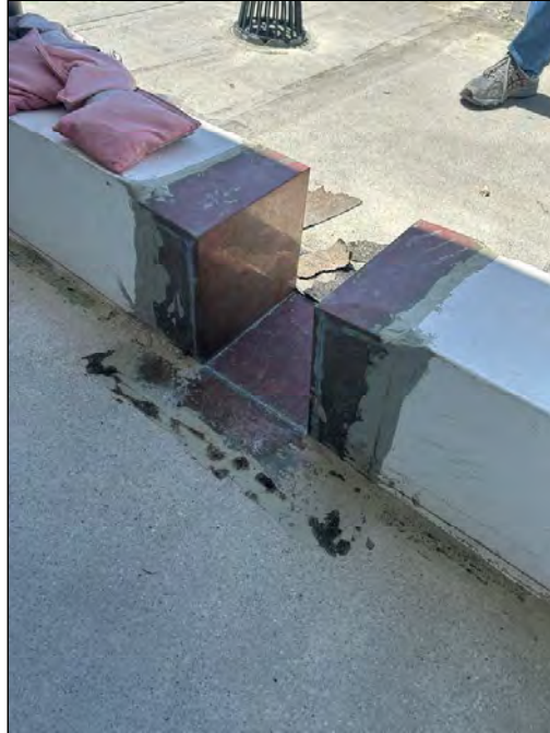
13 - Improper slope at roof. restraining the water flow.
