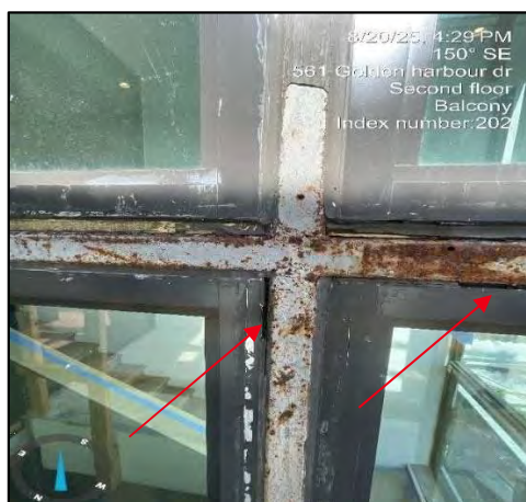
Photo 202 –Missing Sealants at staircase landing at the second floor.
