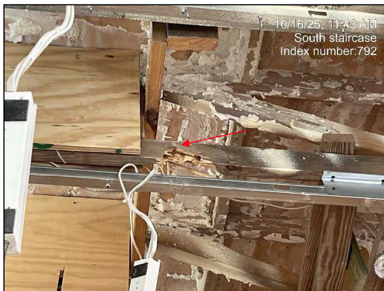
Photo TC_00792 – Damaged/broken truss member at south staircase ceiling (3 rd level).
