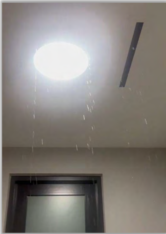
Figure 1: Water leaking from light fixture and air conditioning diffuser in laundry room.
