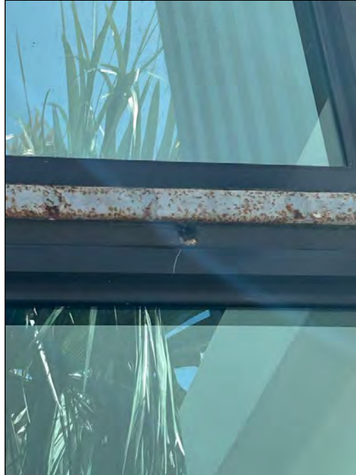
27 - Observed hole along sealant joint.
