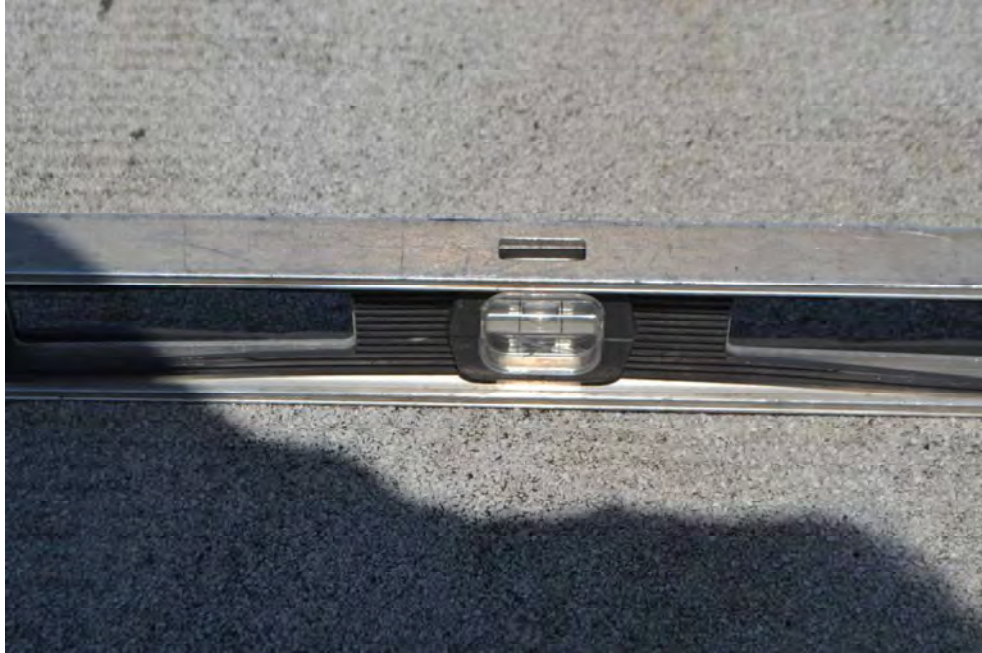
Figure 25) Exemplar view showing the front third floor roof with improper slope.
