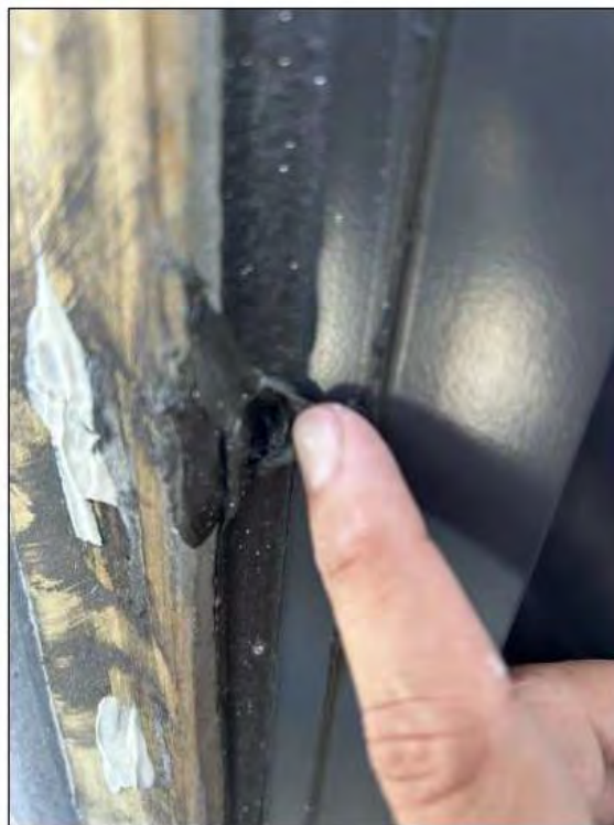
ECS Photo 23: General view of damaged sealant at window (exterior).
