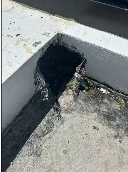
9 - Roofing membrane to be repaired.
