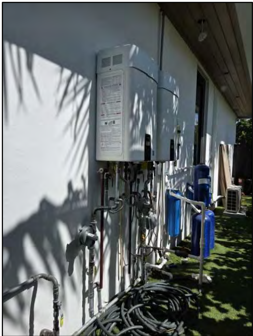
Gas-fired instant water heaters
