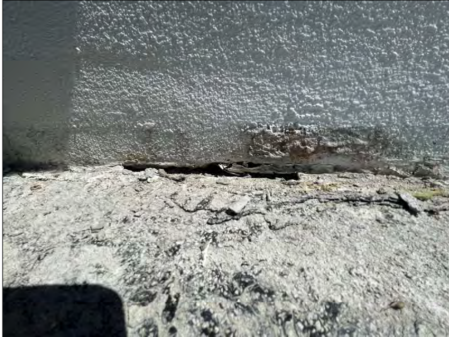
11 - Not signs of proper flashing at roofing membrane.
