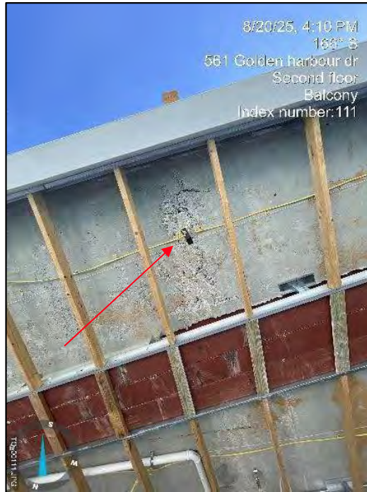
Photo 111 – Honeycombing at the overhead ceiling slab at the outdoor living area at the first floor.
