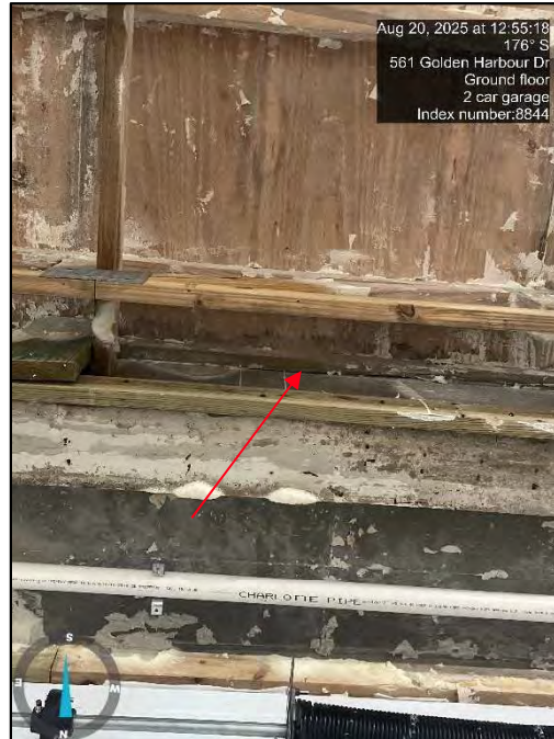
Photo 8842 – Signs of water intrusion from the ceiling in west garage at first floor.
