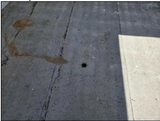
BBQ Area drain missing grate/strainer assembly
