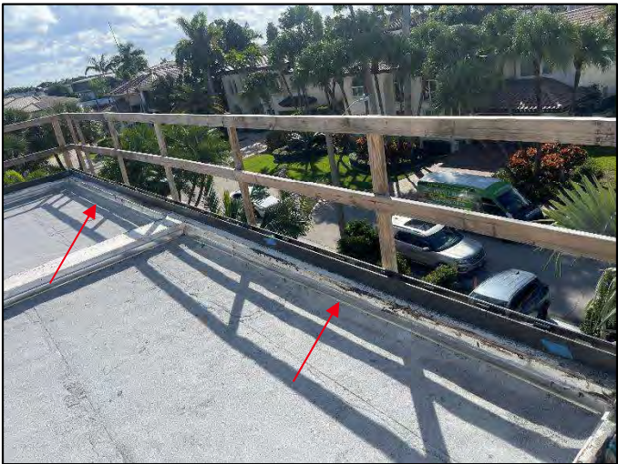
Photo 5638: No scupper was provided at the curb of the South terrace at third floor.
