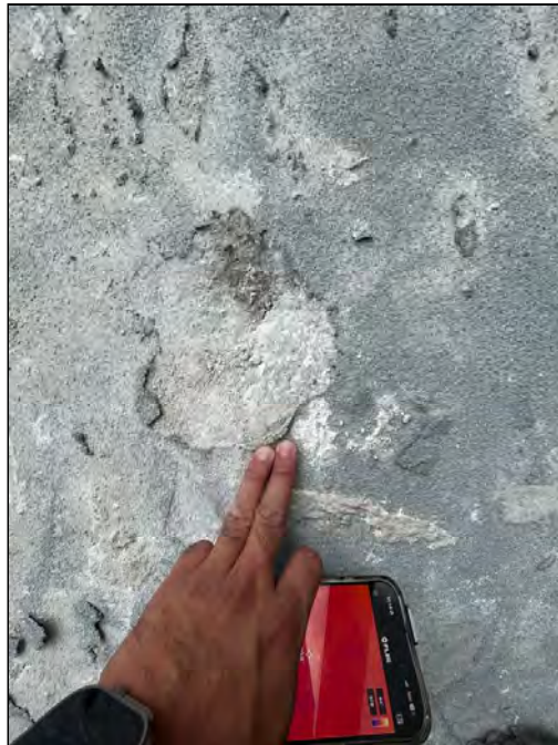
16 - Waterproofing system not properly adhered to the substrate.
