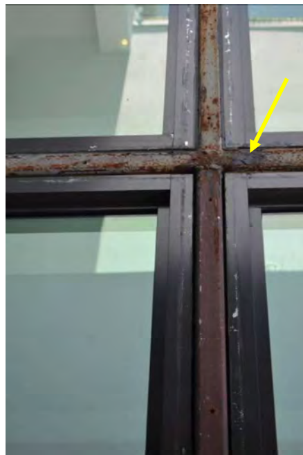
Figure 4) Exemplar view of corrosion observed to the steel tube framing at the exterior wall of the main stair.
