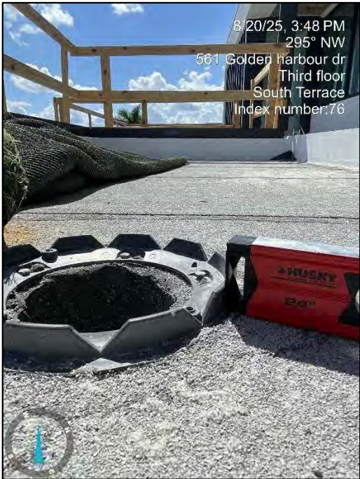
Photo 76: The slope of the roof is away from the drain at South-East Terrace on the 3 rd Floor.
