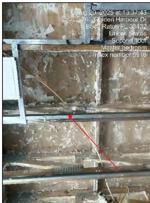
Photo 8916 – Water intrusion from the overhead slab in master bedroom at second floor.
