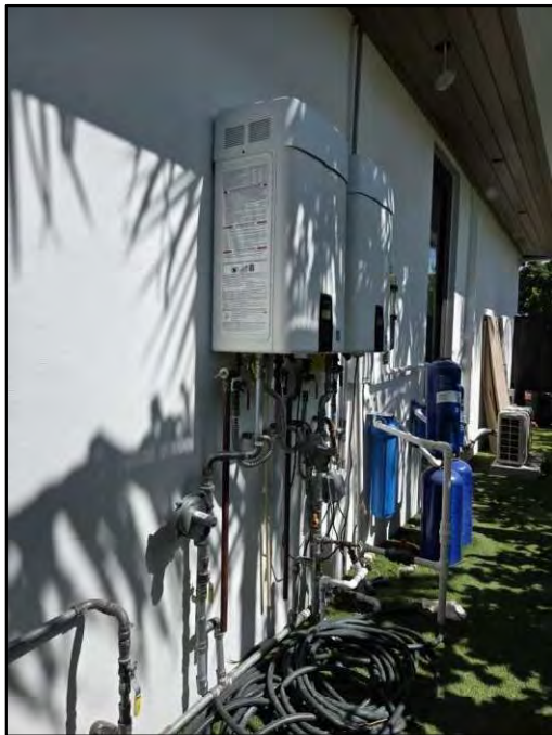
Gas-fired instant water heaters exposed to coastal environment
