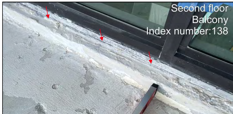
Photo 138: Mortar bed in contact with fixed glass door frame at the second-floor balcony area adjacent to the living room.
