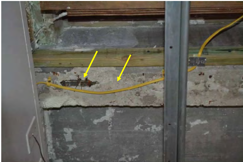
Figure 50) View of spalled concrete and inadequate concrete strength at a beam above the garage.
