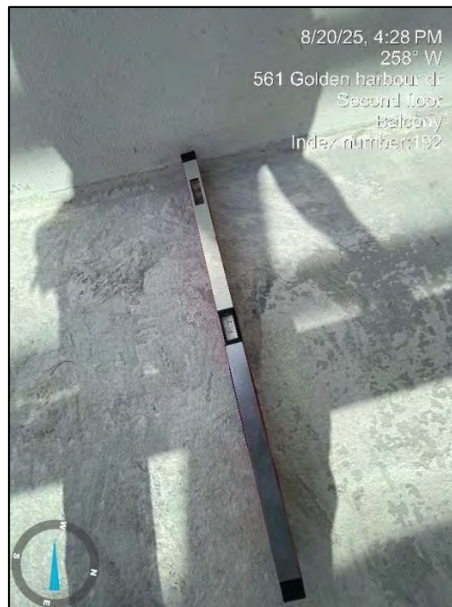
Photo 192: Second Floor Balcony – General view of the south balcony adjacent to the office without any slope.
