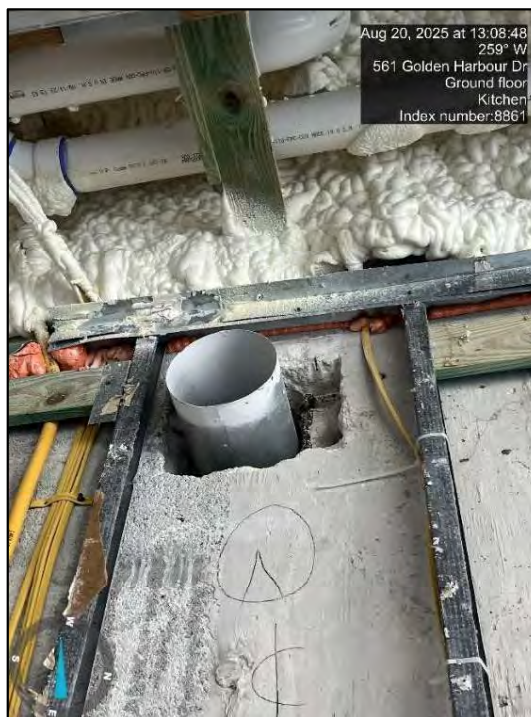
Photo 8861 – Pipe penetration at the column at Kitchen, not shown on structural drawings.
