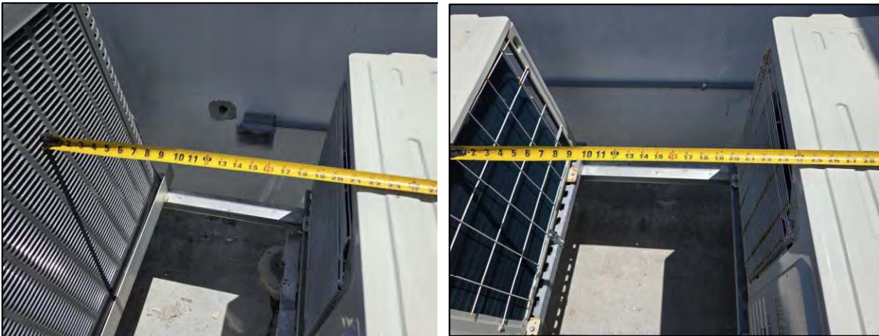
Typical conditions of insufficient clearance around equipment.
