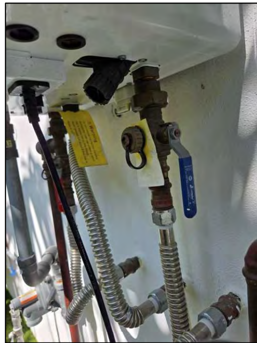
Water supply connection to the water heater missing required check valve
