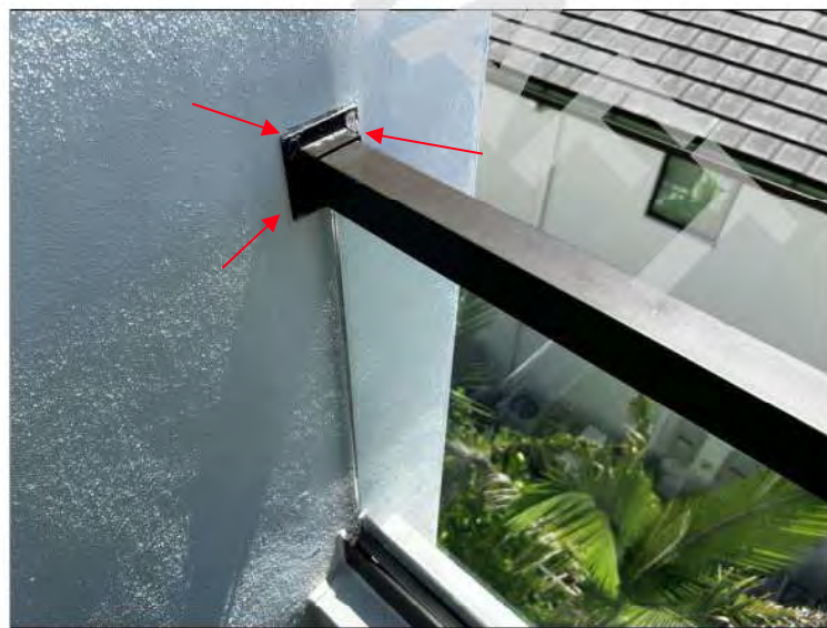
ECS Photo – Unsealed and missing fasteners at the balcony railing.
