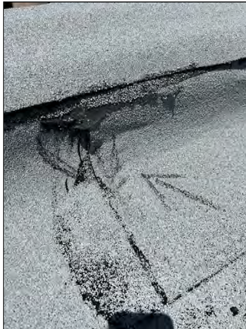
2 - Roof membrane was marked for remediation.
