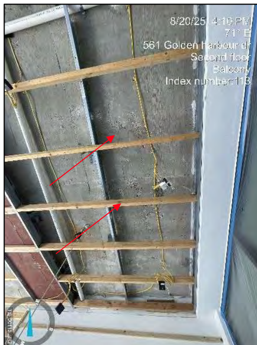
Photo 113 – Honeycombing at the overhead ceiling slab at the outdoor living area at the first floor.
