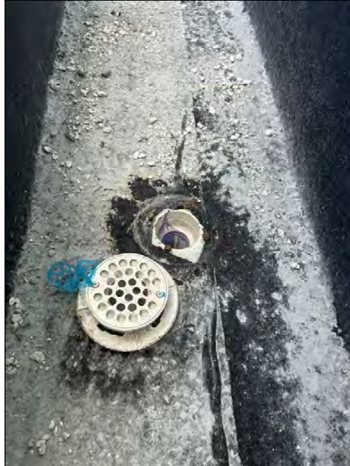
3 - Drain body without proper level.
