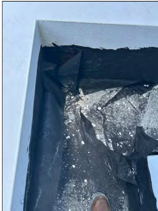
4 - No termination bar or detailing observed for the waterproofing system at planter.
