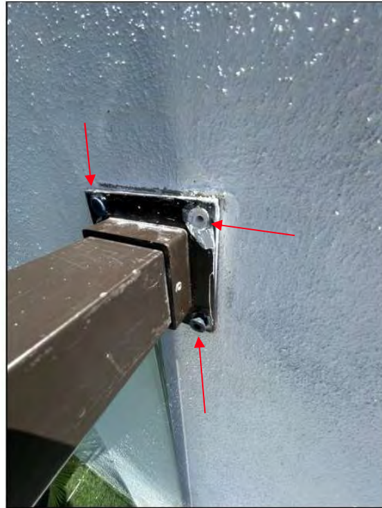
ECS Photo 12 – Unsealed and missing fasteners.
