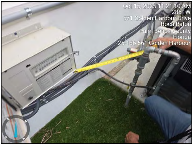
Pool heater regulator within 3 feet of control panel
