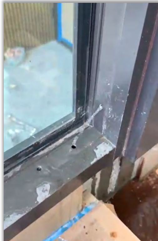
Figure 2: Water spouting from window frame in main staircase after screw removal.
