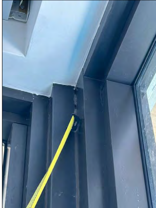
25 - Sealant bead with visible voids and holes.
