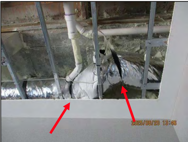
Typical condition of flexible duct with sharp bend and compressed insulation, Bedroom 1.
