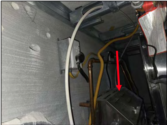
Steam generator equipment installed behind the gas burning cooking equipment.
