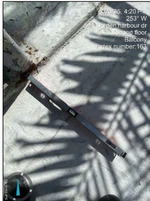
Photo 163: Second Floor Balcony – General view of the north balcony adjacent to the Her bathroom without any slope.
