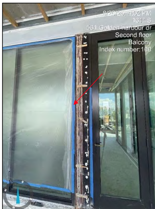
Photo 100 – Corroded metal column at balcony at the second floor.
