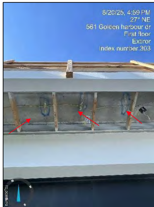
Photo 303 – Multiple cracks at the concrete ceiling slab at the Southwest corner of the office – 2 nd level.
