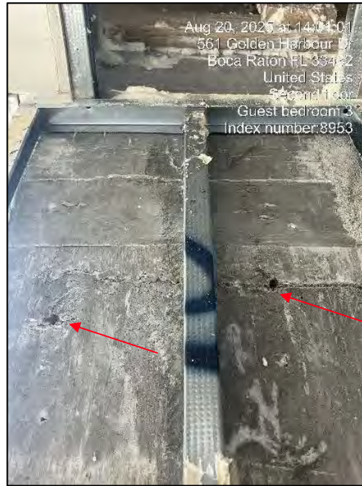
Photo 8953 – Corroded metal is visible at wall in Guest bedroom #3 at the 2 nd Floor.
