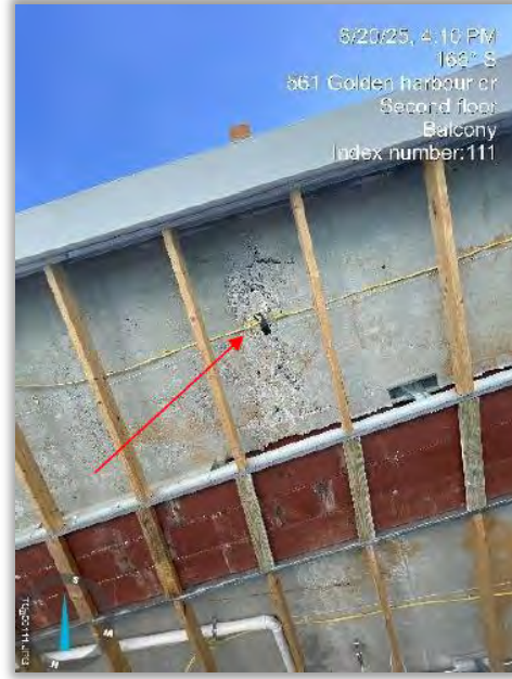
Figure 8: honeycombing concrete on balcony slab and exposed rusting rebar
