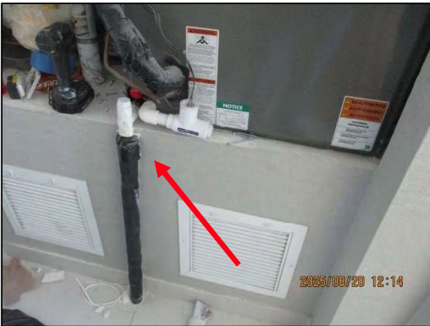
AHU #2 condensate drainage line missing trap
