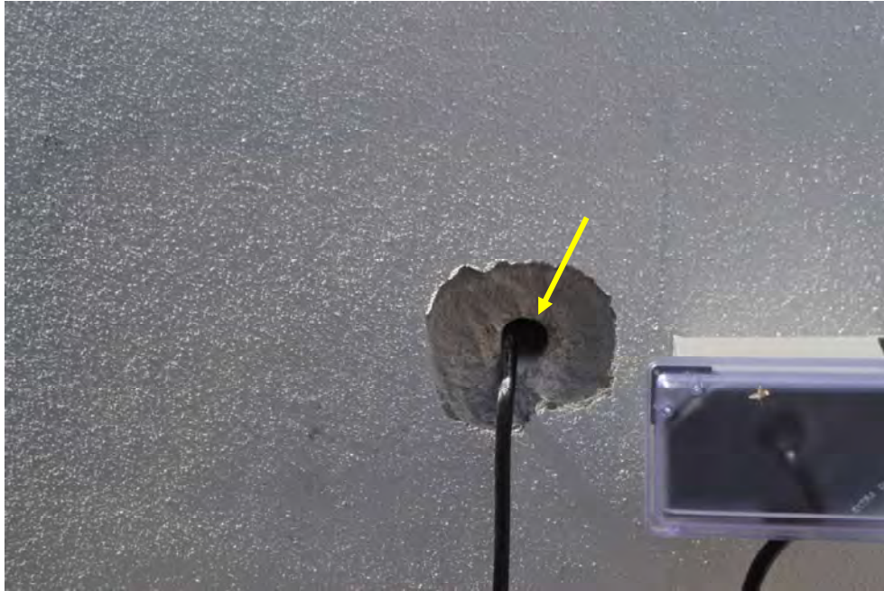
Figure 19) View of a wall opening at a wire penetration at the outdoor mechanical area.
