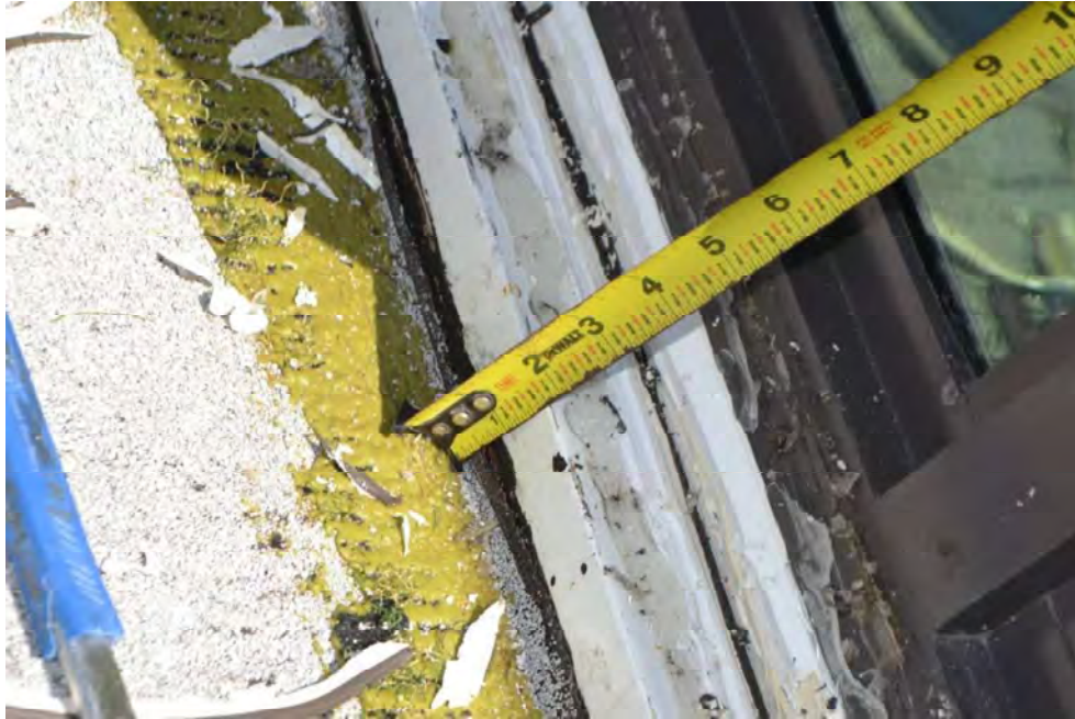
Figure 23) Exemplar view showing inadequate flashing height at the front third floor roof.
