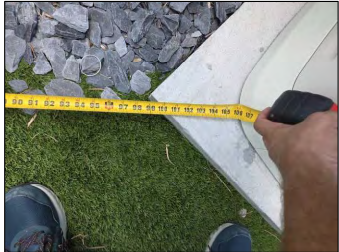
Equipment within 10 feet of building opening
