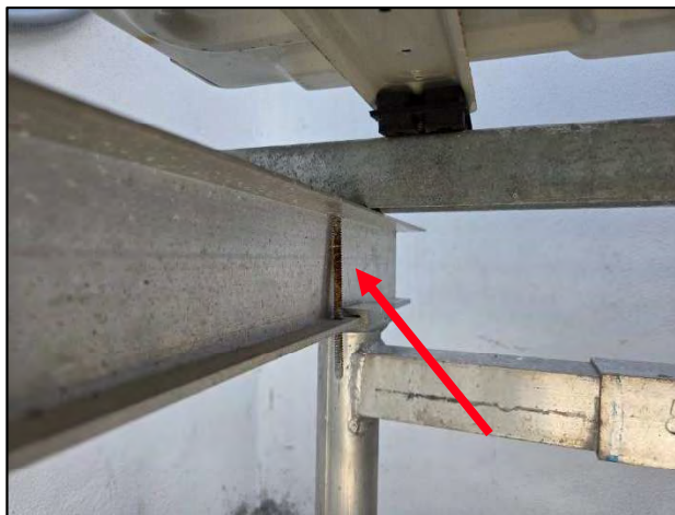
Corroded galvanized steel anchor in contact with aluminum equipment stand
