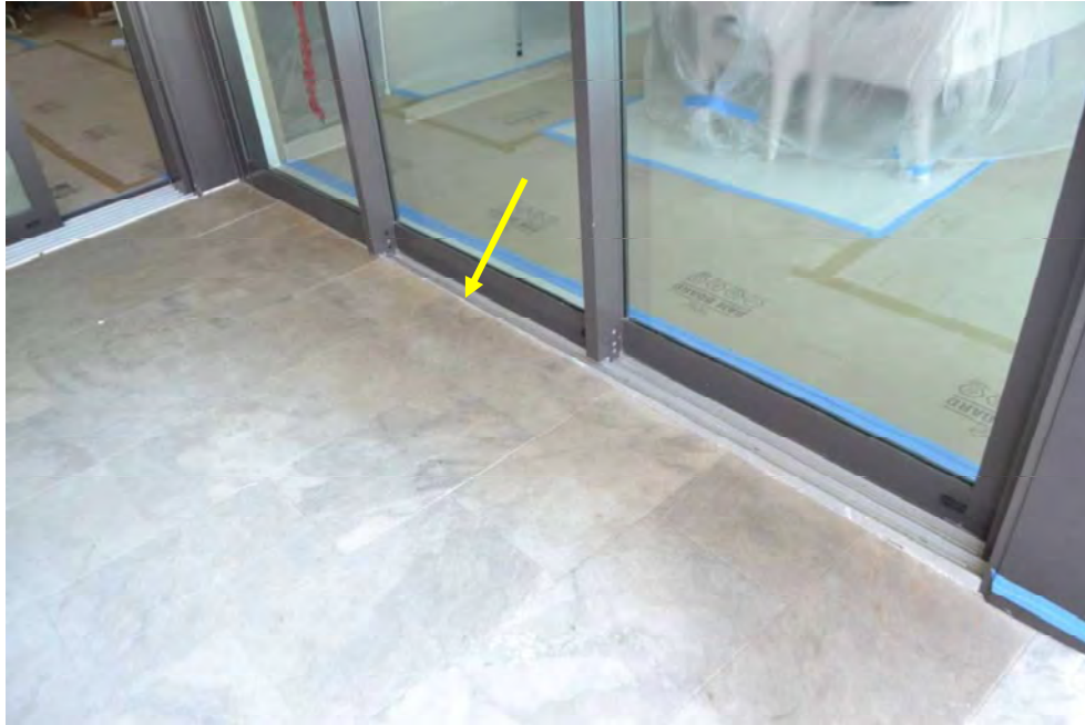
Figure 57) View showing pavers covering the slider track weep holes at the rear porch.
