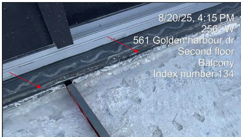
Photo 134: Mortar bed in contact with sliding glass door frame at the second-floor balcony area adjacent to the guest bedroom #1.
