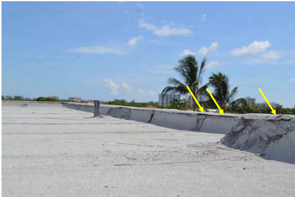
Figure 28) Exemplar view of apparent openings observed in the upper roof covering along the perimeter curb.
