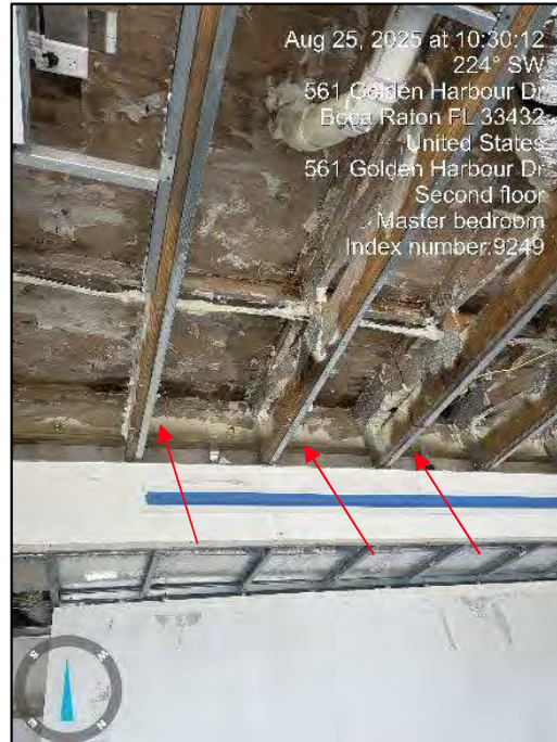
Photo 9249 – Water intrusion at the overhead slab in master bedroom at second floor.
