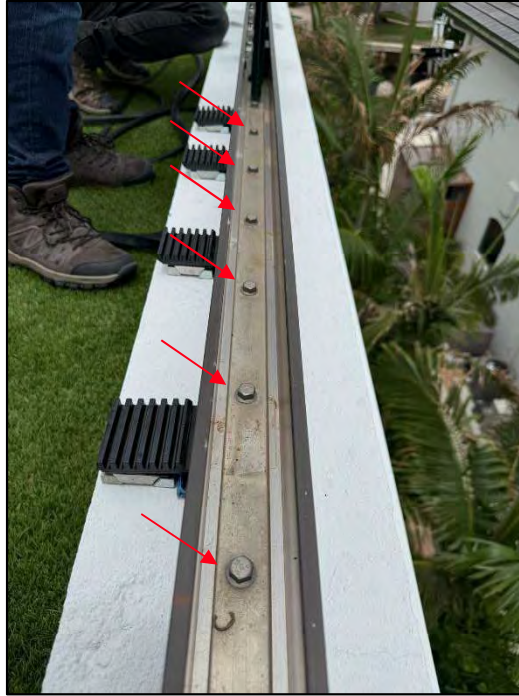
561-6.5.25-Pic #13 – Fasteners at the base of railing system were not provided with sealant.
