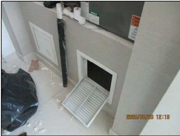
Return air plenum box for AHU #1 and #2
