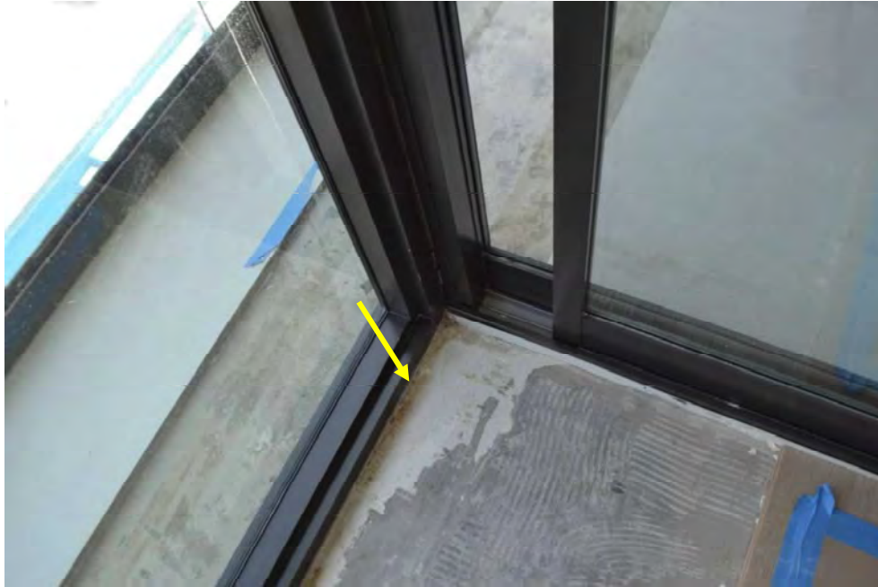
Figure 37) Exemplar view of water staining observed to the concrete in the master bedroom near the exterior windows.
