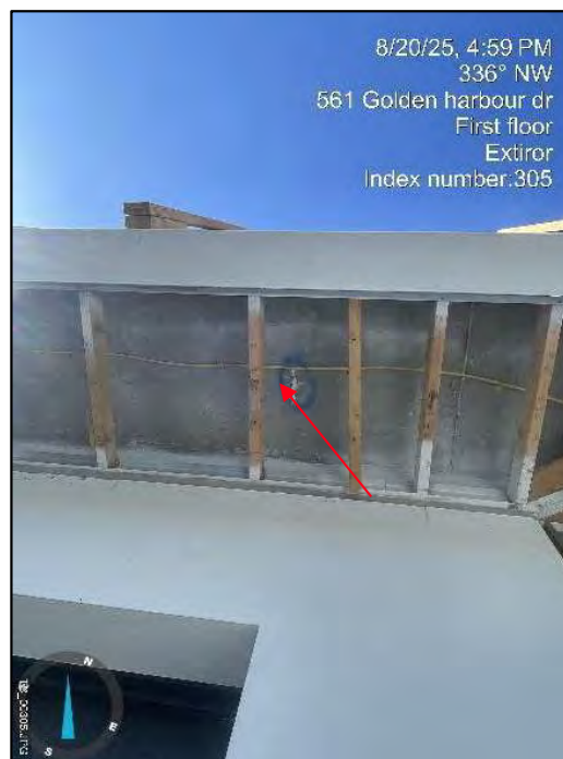
Photo 305 – Multiple cracks at the concrete ceiling slab at the Southwest corner of the office – 2 nd level.
