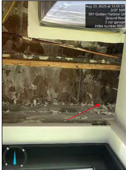
Photo 8852 – Signs of water intrusion from the ceiling in east garage at first floor.
