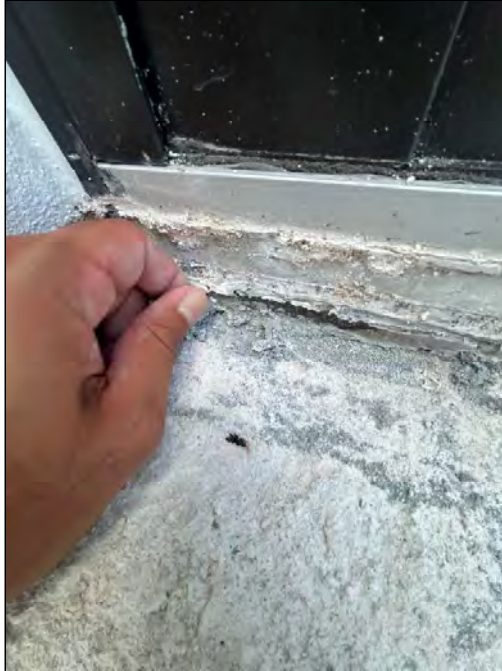
17 - Sealant gap between window frame and substrate.
