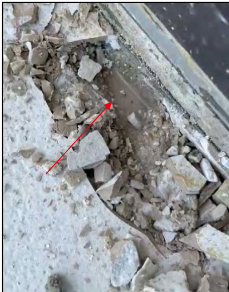
Photo 561 – 6.9.25 – Video #1 Still: Second Floor Balcony – Showing water standing below floor finishes during demolition adjacent to window wall.
