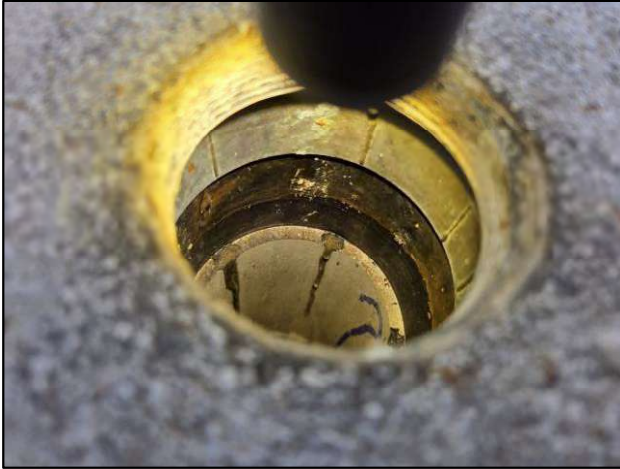
Opening at roofing system smaller than drain outlet and obstructing water flow.
