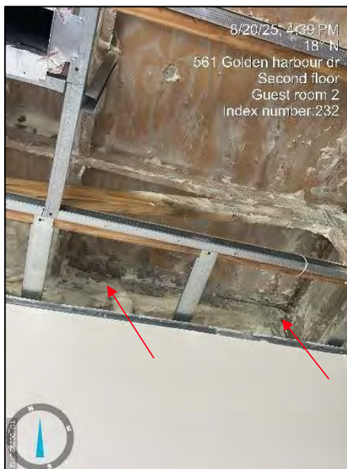
Photo 232 – Water intrusion at the overhead slab in guest bedroom#2 at second floor.
