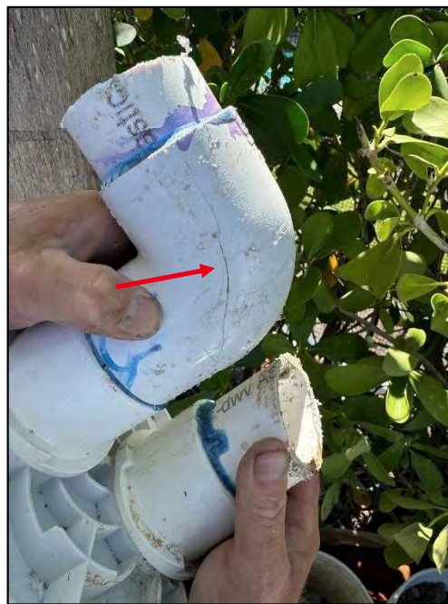
Cracked found in the connected pipe fitting
