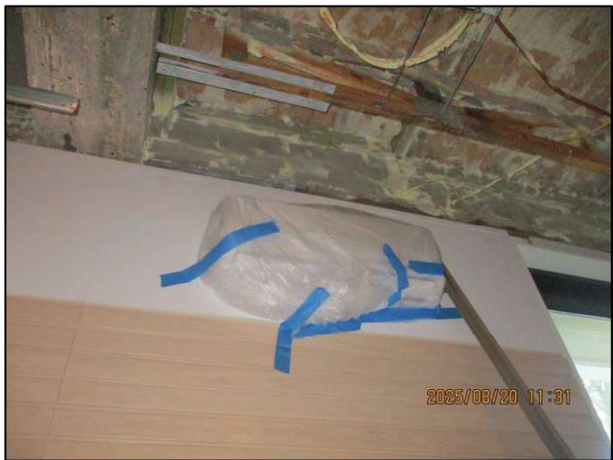
Air handler for the mini split system in the Garage
