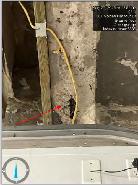
Figure 7: crumbling concrete over exposed rusting rebar
