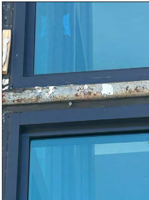
26 - Screws were installed directly through sealant joints.
