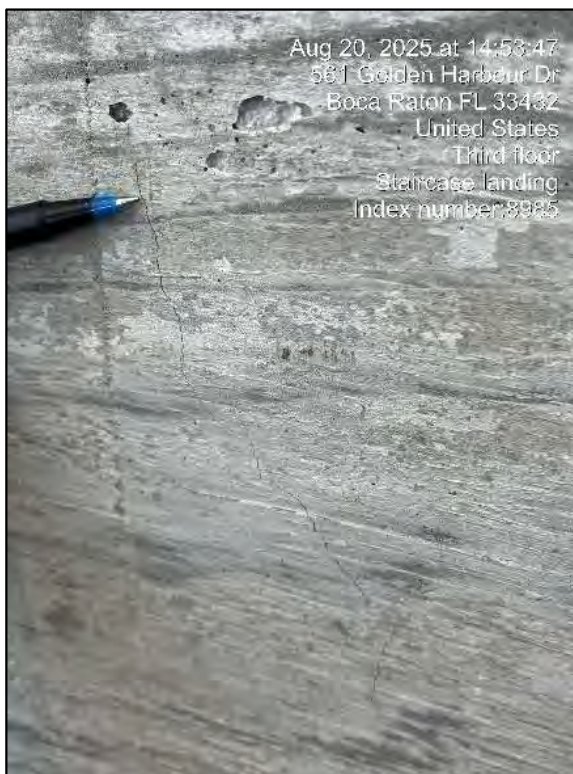
Photo 8985 – Crack at the beam at Staircase landing – 3 rd Floor.
