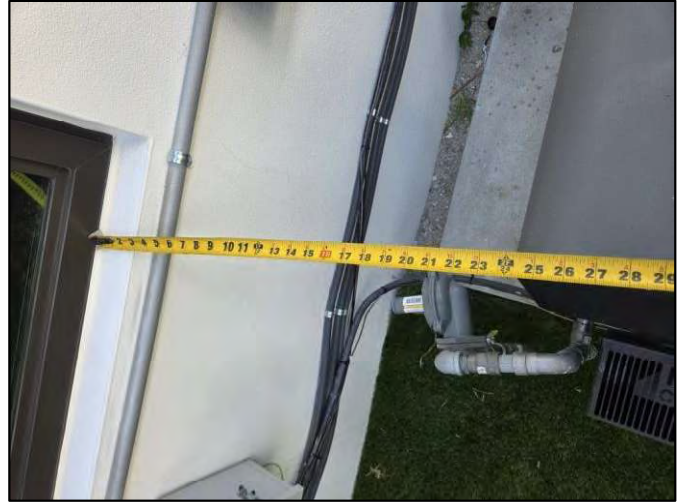
Gas-fired heater installed within 4 feet of the operable window.
