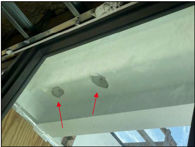
Photo 5593 – Penetrations made in the slab at second-floor walkway (at the south side -front portion of the residence) in order to drain ponding water.
