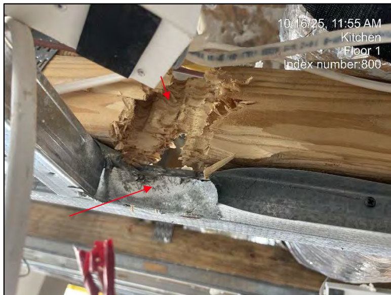
Photo TC_00800 – Damaged/broken truss member is visible at kitchen at Level-2.
