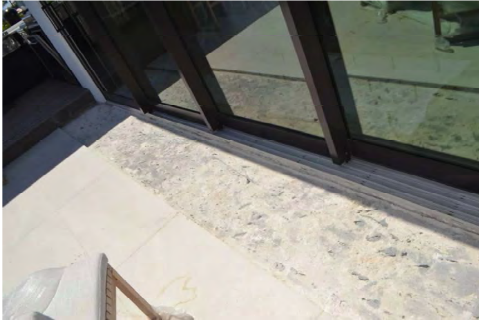
Figure 15) Exemplar view of removed pavers at the third floor rear balcony. Note pavers installed above the slider track weep holes in some locations.
