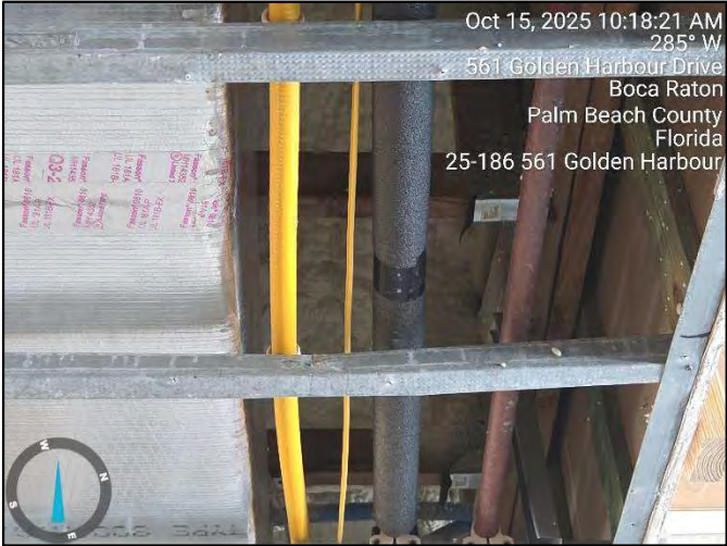
Installation of the CSST missing protection shield
