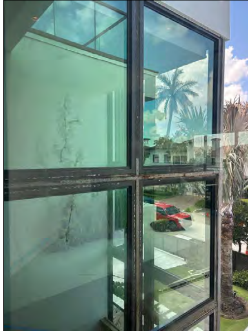
19 - Windows observed missing backer rod and sealant installation.
