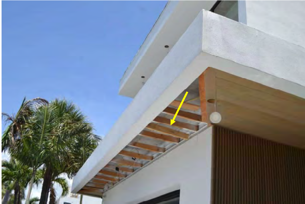
Figure 53) View showing the reportedly water damaged soffit finish removed at the garage.
