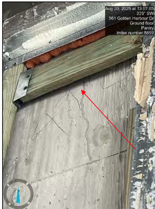
Photo 8859 - Water intrusion coming from the exterior at the column in the kitchen pantry at ground/first floor.
