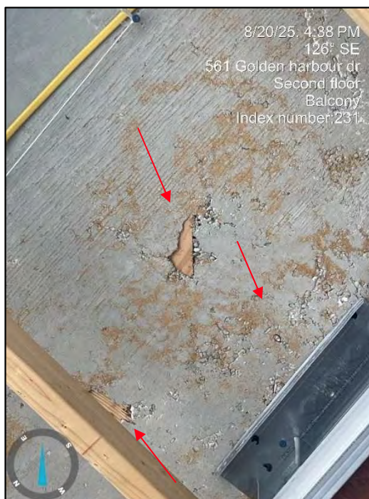
Photo 231 – Honeycombing and wood embedded in the ceiling slab at the balcony at second floor.
