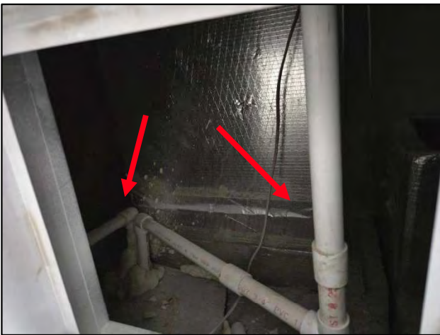
AHU #4 PVC condensate drain within return air plenum.
