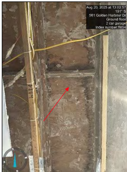
Photo 8854 – Signs of water intrusion from the ceiling in east garage at first floor.
