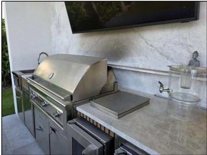
Outdoor, gas-burning cooking equipment at the backyard areas
