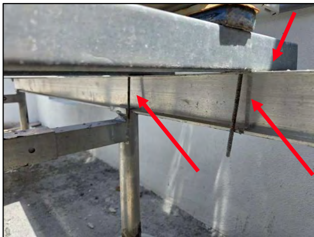
Galvanized steel Unistrut and anchors in contact with aluminum stand, typical dissimilar metals in contact
