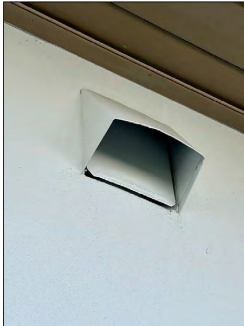
34 - Vent observed without sealant installed.
