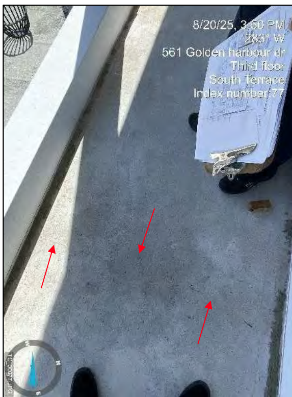
Photo 77 – Crack at the floor slab at South Terrace – 3 rd Floor.
