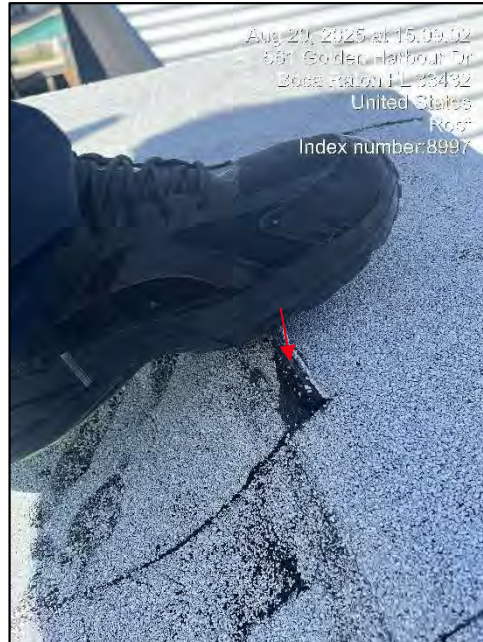
Photo 8997: View of loose / debonded roofing membrane. at the roof curb.
