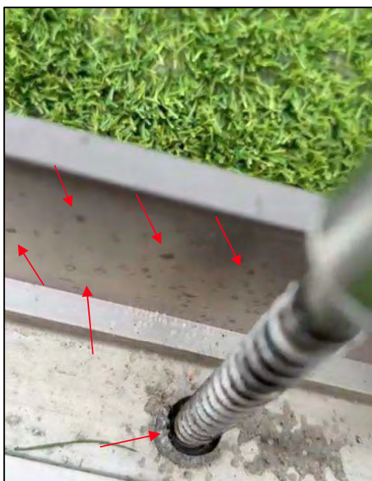
561-6.5.25- Video#1 Still 2 – Showing water droplets expelled during removal of unsealed fastener from railing system base channel.
