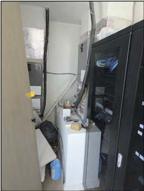
Return air plenum box for AHU #1 and #2
