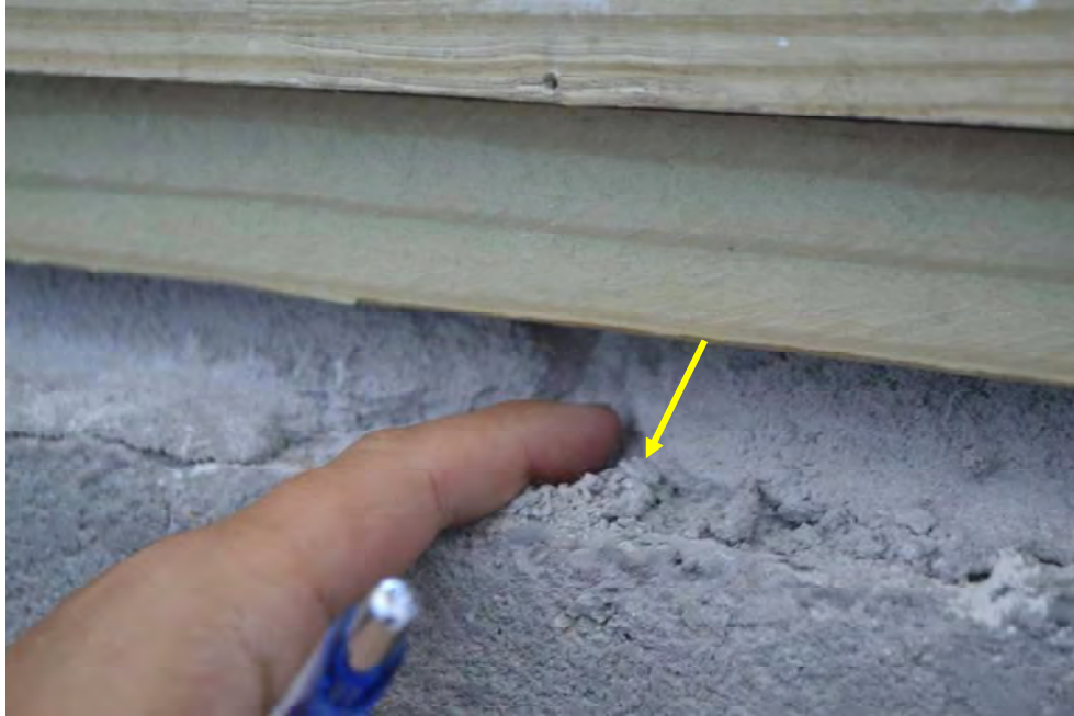
Figure 11) Close-up view of low-strength grout installed between the window buck and concrete beam at the stair to the third floor.
