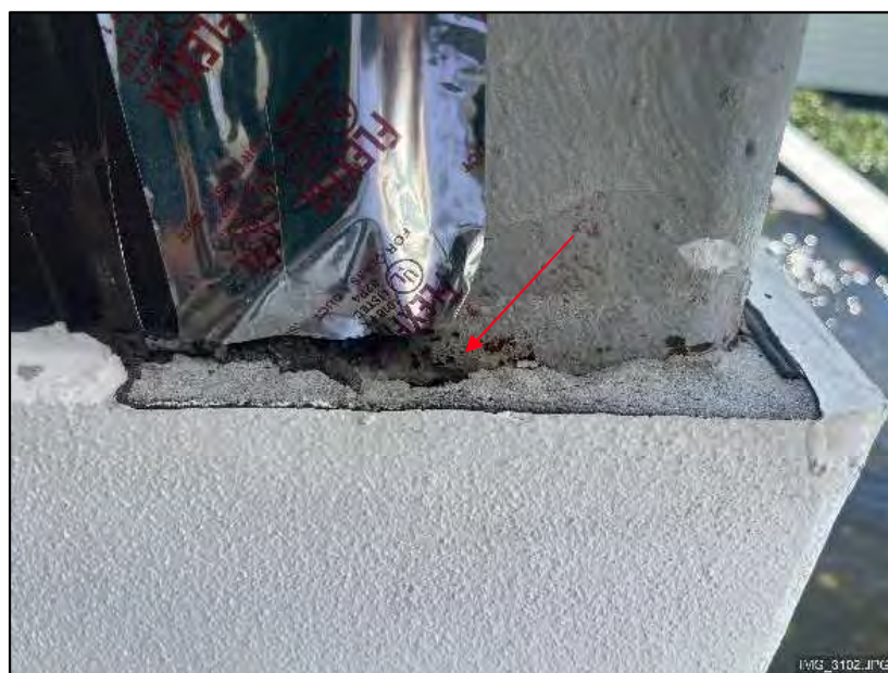
Photo 3102 – Corroded metal column potentially embedded in staircase landing floor slab at the second floor.
