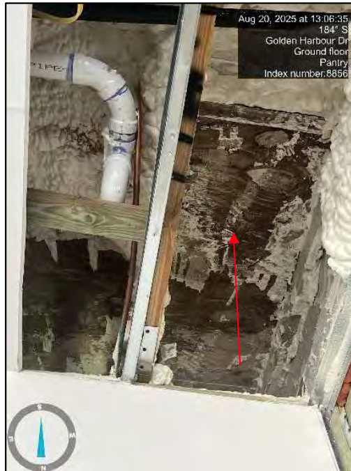
Photo 8856 – Water intrusion from the ceiling in pantry at first floor.
