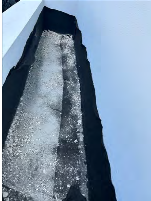
5 - Inconsistent waterproofing membrane applied.
