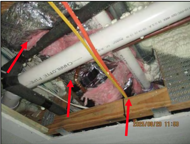
Typical condition of flexible ducts squeezed between floor beams, joists, and building systems, Laundry Room.
