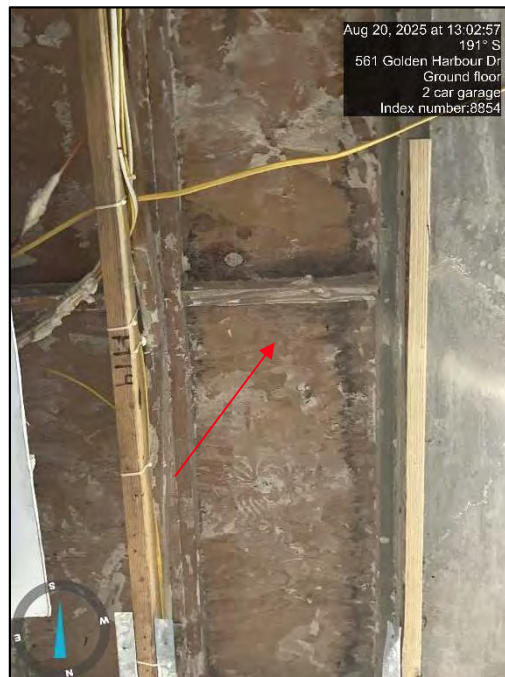
Photo 8854 – Signs of water intrusion from the ceiling in west garage at first floor.
