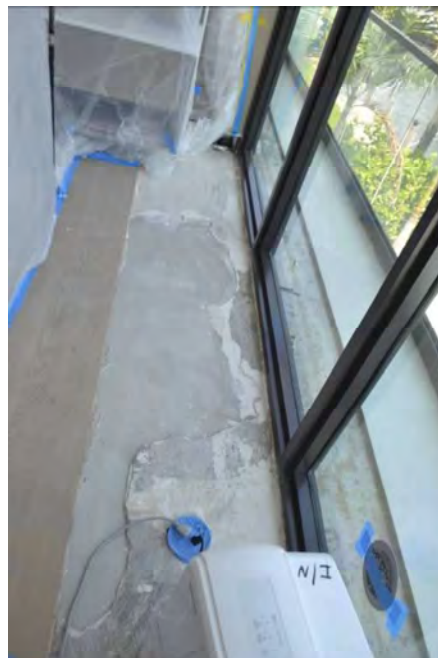
Figure 36) View showing the reportedly water damaged wood flooring removed in the master bedroom along the exterior windows.
