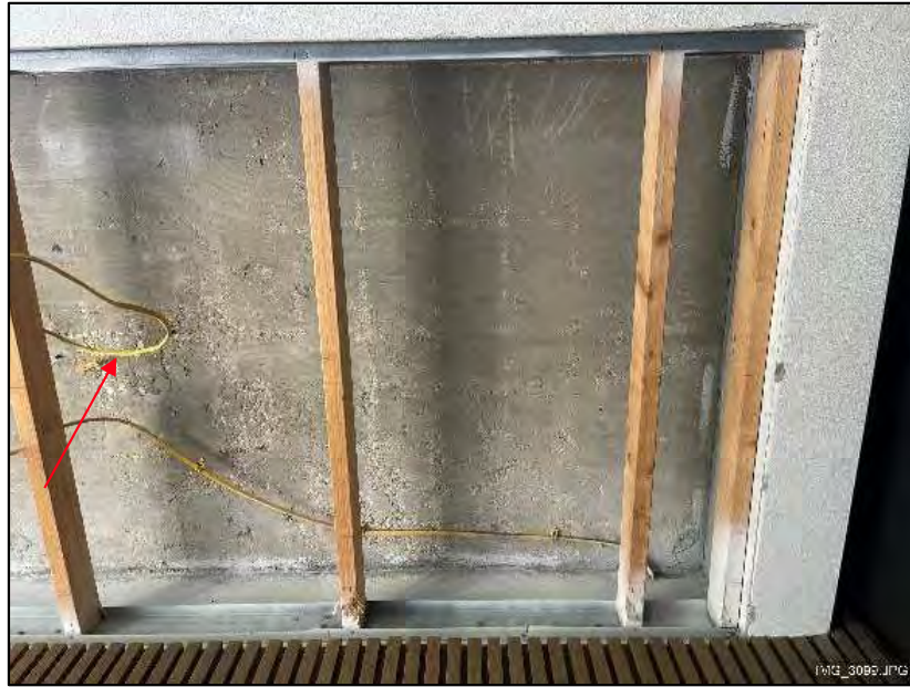
Photo 3099 – Honeycombing at the overhead ceiling slab at the main entrance adjacent to the garage area at the first floor.
