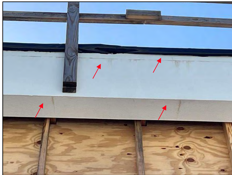
Photo 6095 – Cracks in Stucco at exterior parapet wall at Level-3.
