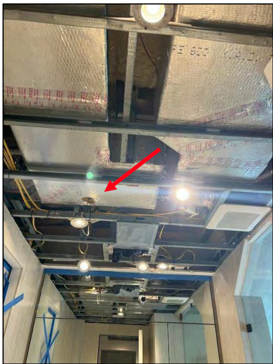
Opening in duct above Master Bathroom due to light fixture installation (photograph provided by renovation contractor)
