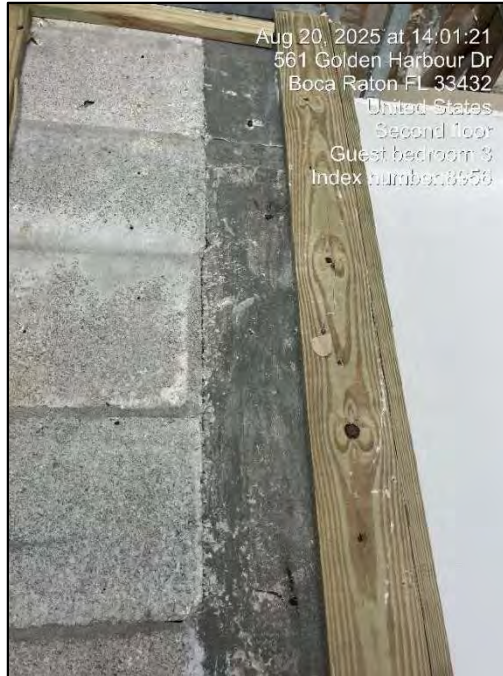
Photo 8956 – Crack in joint between masonry wall and column at the guest bedroom #3 on second level.
