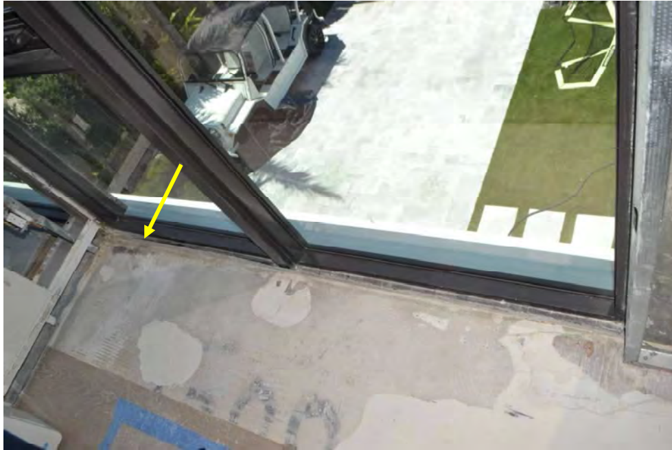
Figure 45) View of water staining observed to the concrete in the son's bedroom.
