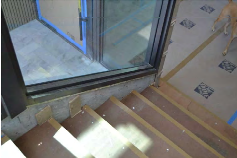
Figure 3) View of reported water damaged removed wall finish at the main stair.
