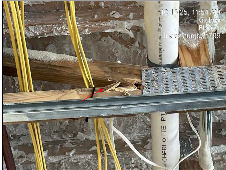
Photo TC_00799 – Damaged/broken truss member is visible at kitchen at Level-2.
