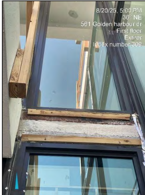
Photo 309 – Corroded metal beam/mullion at second floor slab above the main door.
