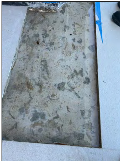
32 - Tile installed over concrete without waterproofing membrane,
