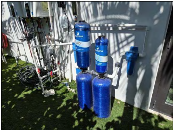
Whole-house water filtration system
