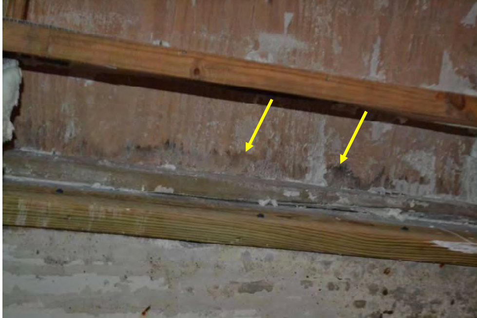
Figure 51) Exemplar view of water staining observed to the floor sheathing above the garage near the exterior planter.
