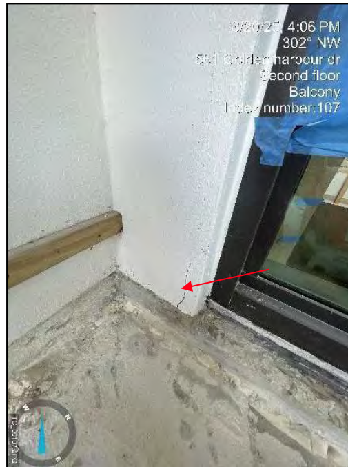
Photo 107 – Delaminated stucco at the exterior wall of the master bedroom at the second level.
