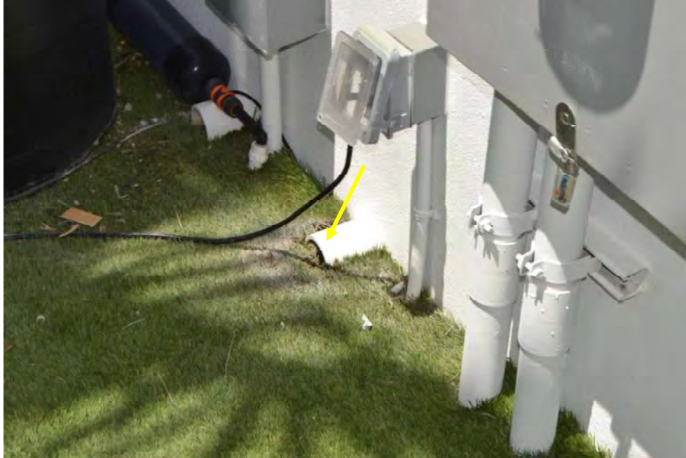
Figure 63) View showing exterior grade above a roof drain outlet at right elevation of the home.
