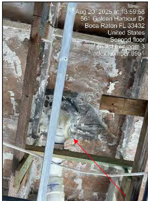
Photo 8951 – Signs of water intrusion adjacent to the pipe penetration at the overhead slab in guest bedroom #1 at second floor.
