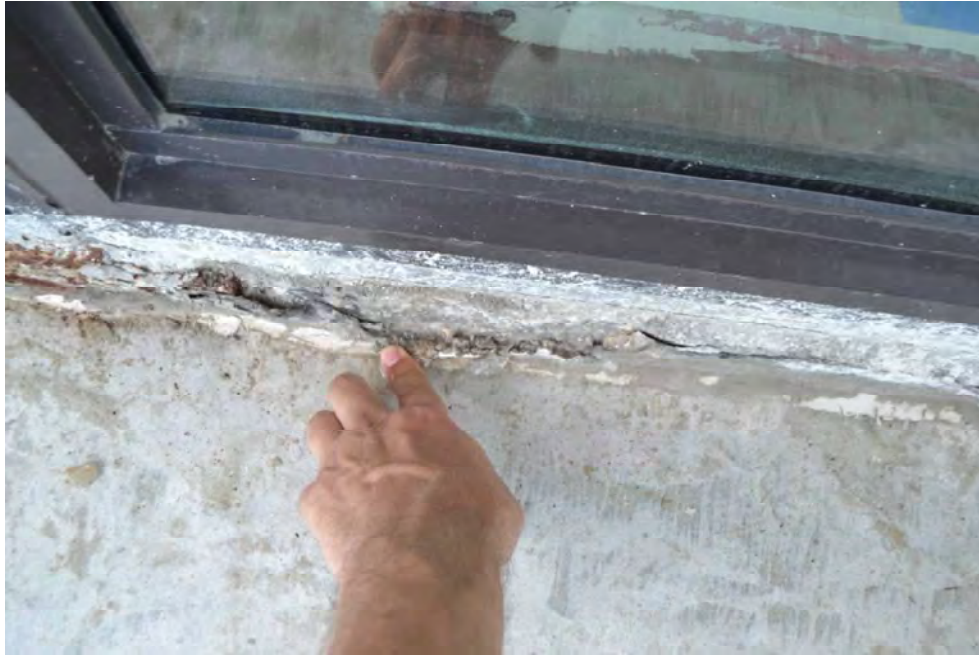
Figure 35) View showing no waterproofing or flashing observed at the second floor rear balcony.
