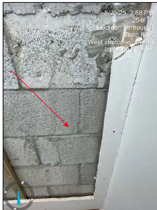
Photo 98 – Crack in masonry wall at the west staircase landing at the third floor.
