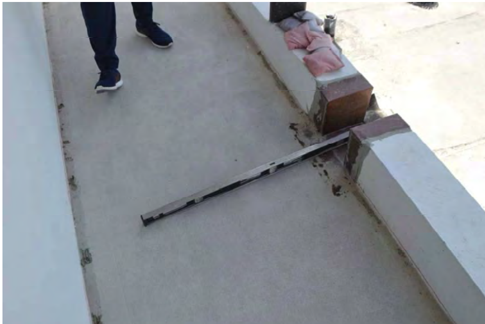
Figure 24) View showing the front third floor balcony with improper slope.
