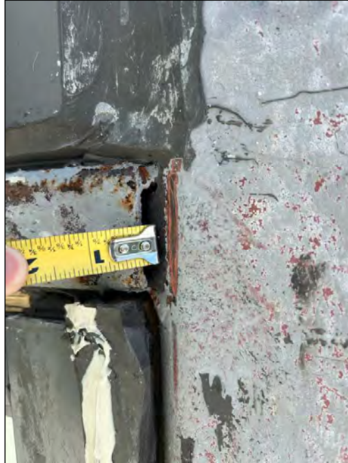
7 - Gap at windows assembly, to be properly detailed.
