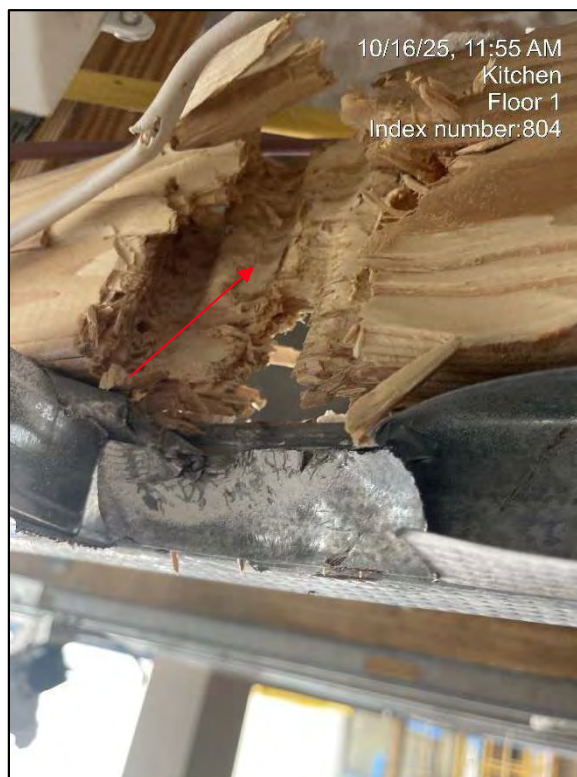
Photo TC_00804 – Damaged/broken truss member is visible at kitchen at Level-2.
