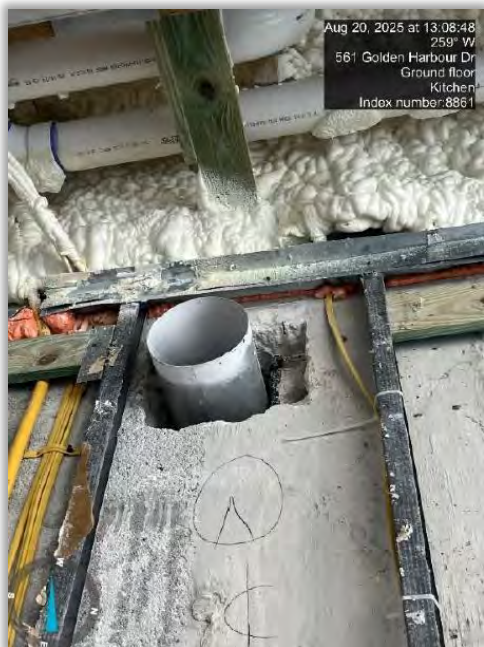
Figure 11: kitchen air vent penetrating structural reinforced concrete column
