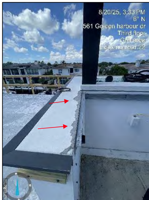
Photo 22 – Delaminated stucco at parapet wall adjacent to Grill area at Level 3.
