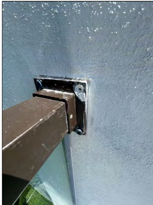
12 - Railing system observed missing screws.
