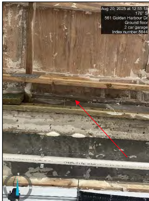
Photo 8844 – Signs of water intrusion from the overhead slab in east garage at first floor.
