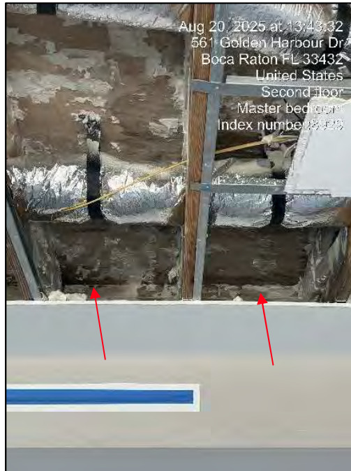
Photo 8929 – Water intrusion from the overhead slab in master bedroom at second floor.
