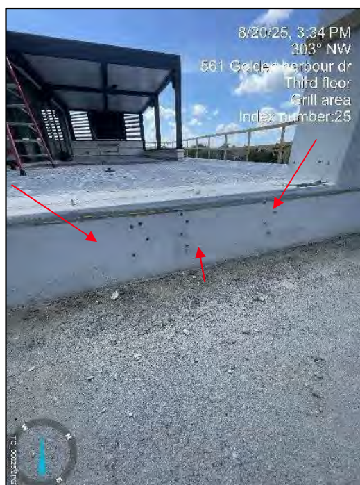
Photo 25 – Stucco cracks at wall adjacent to Grill area at Level 3.
