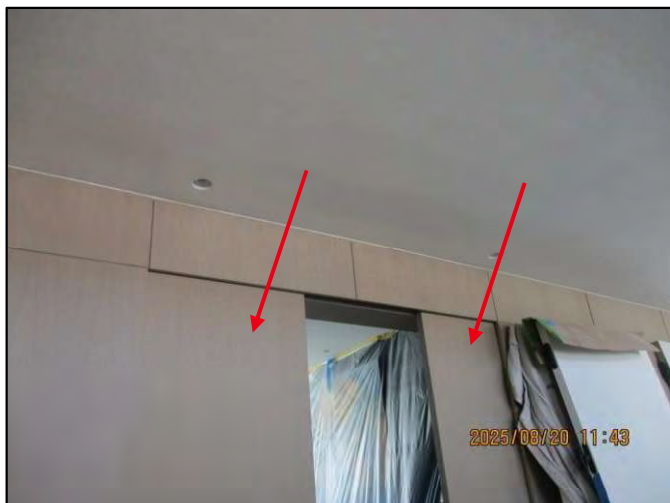
Solid doors installed for Fitness Center and no return air provisions.
