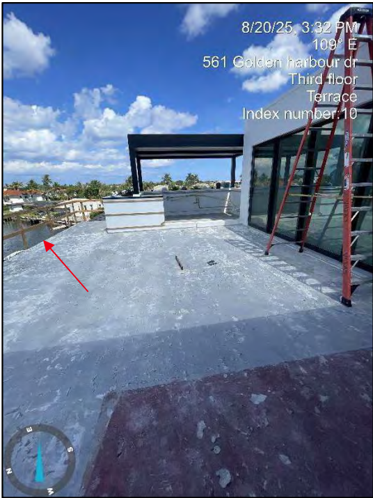
Photo 10: No curb was constructed at North terrace on third floor as specified on sheet P-03.
