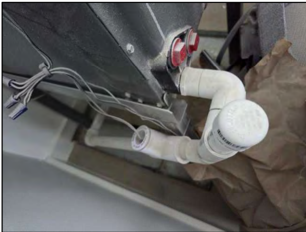
AHU #3 condensate drainage line missing trap
