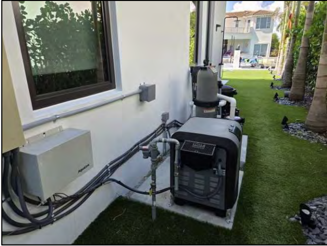
Pool/Spa gas-fired heater equipment located near operable window.
