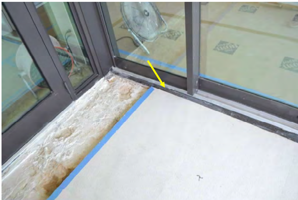
Figure 32) Exemplar view showing pavers installed above the lower window frame at the second floor rear balcony.
