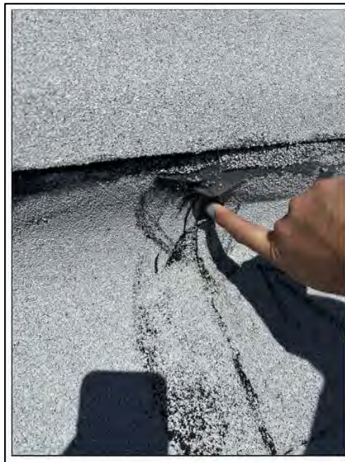
ECS Photo 1: View of unadhered roofing membrane.
