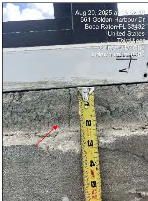
Photo 8983 – Fixed glass window with excessive gap between framing and structural substrate at sill at third level southwest staircase. The arrow shows mortar between substrate and framing of glazing system.
