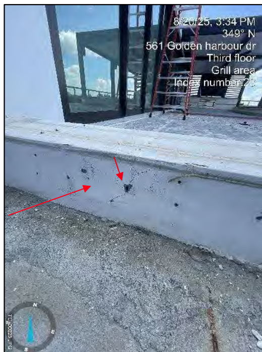
Photo 23 – Stucco crack at parapet wall adjacent to Grill area at Level 3.
