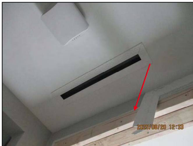
No transfer grille at wall above door.
