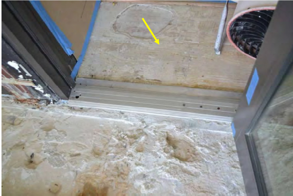
Figure 33) View showing the interior wood flooring removed at the door to the second floor rear balcony reportedly due to water damage.
