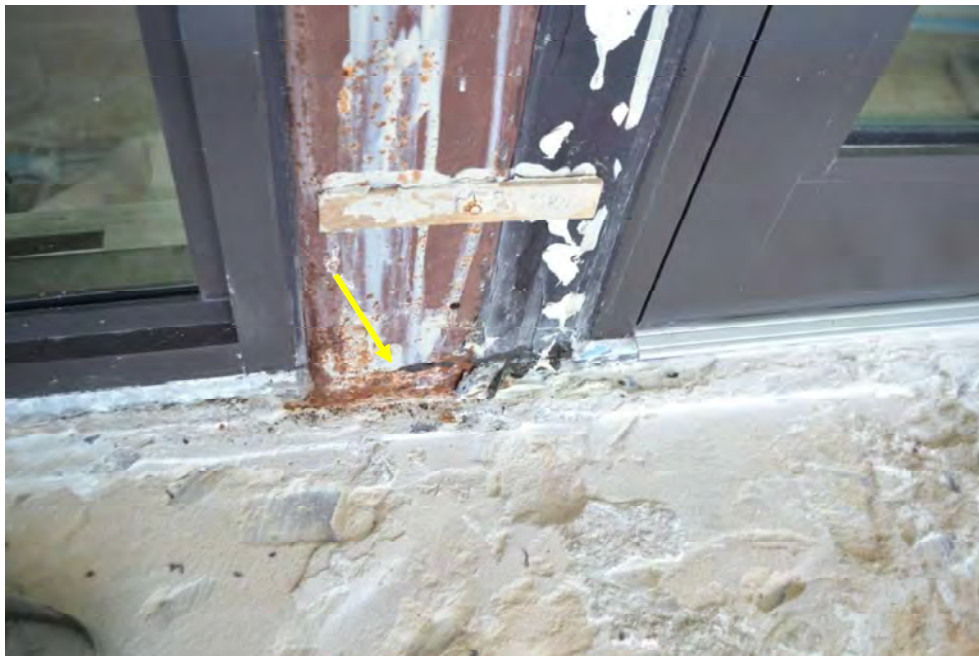
Figure 34) Exemplar view of corrosion observed to the steel column base at the second floor rear balcony.
