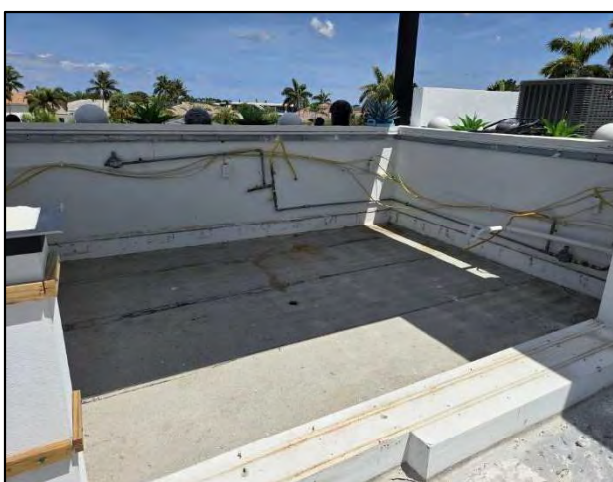
Unsupported gas piping.
