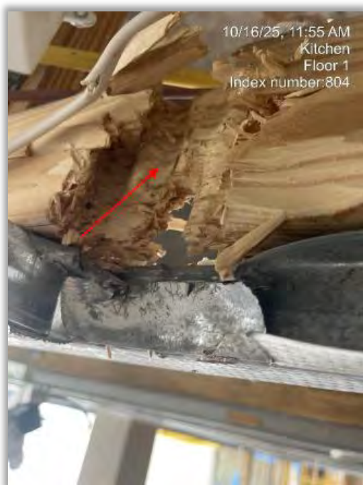
Figure 13: broken roof trusses
